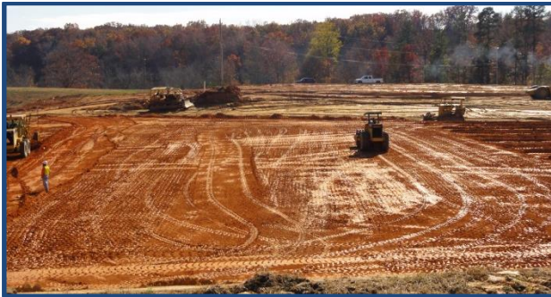
The auxiliary spillway width was increased to handle a larger water flow to protect the dam.
