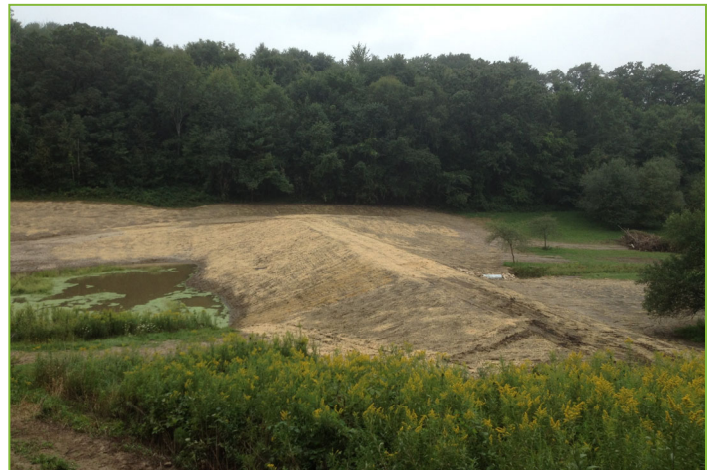
Below: After repairs are done, the embankment and borrow area are seeded and mulched.
