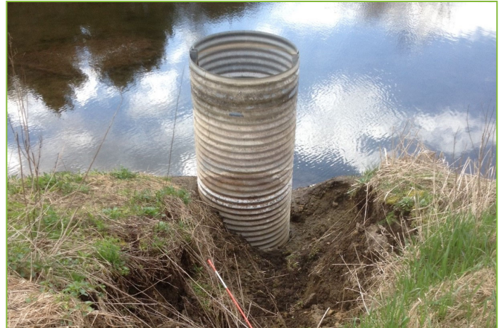
Above: The dam in 2017, showing the gully washing out along the berm. The vertical pipe is set below the top of the berm so water would leave through the pipe rather than over the top of the berm if the horizontal pipe plugged or couldn't carry water fast enough.
