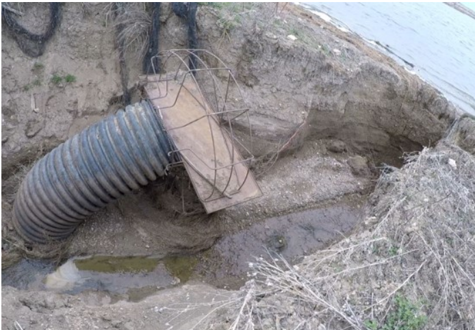
Figure 3. Dam riser failure at Howell Reservoir Dam in Wyoming.
