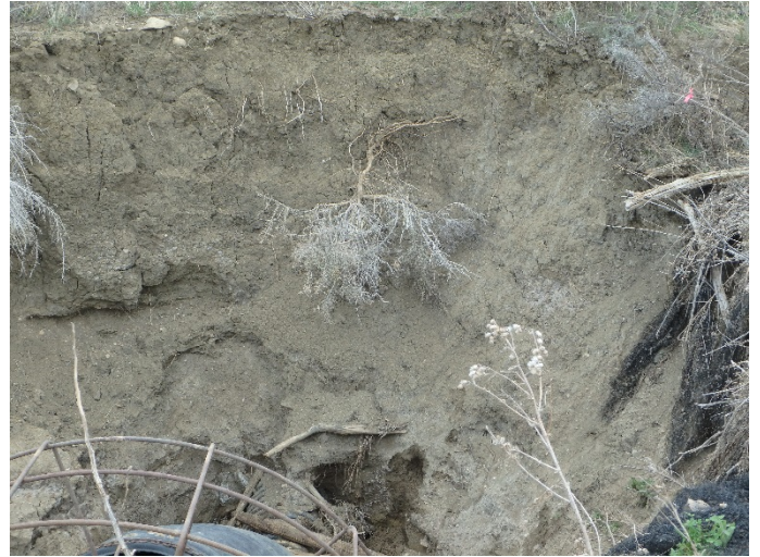
Figure 2. A view into part of the hole created by the failed riser, with the damaged riser at the bottom left.
