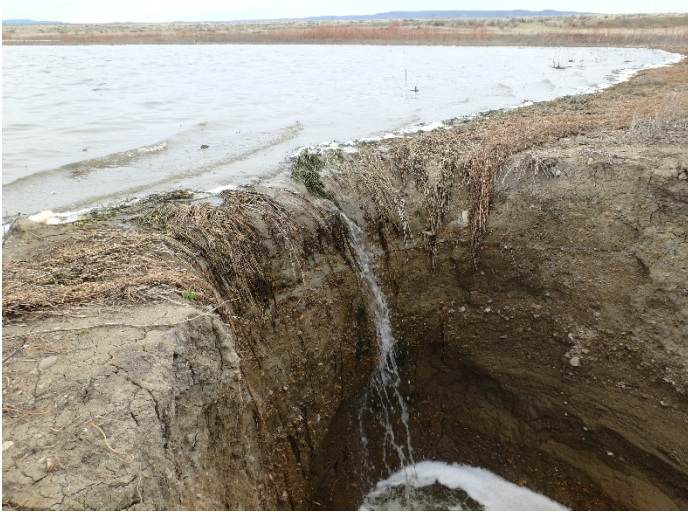
Figure 1. Water from Howell Reservoir Dam pours into the hole created by the riser failure.
