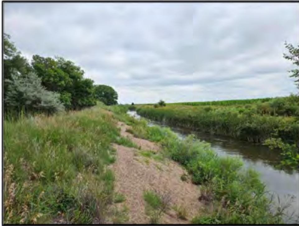
Figure 69. Paxton Hershey Canal: channel overview, Segment 1. Note sediment berm on the left descending bank. View to the northwest. Photograph taken on July 16, 2025.
