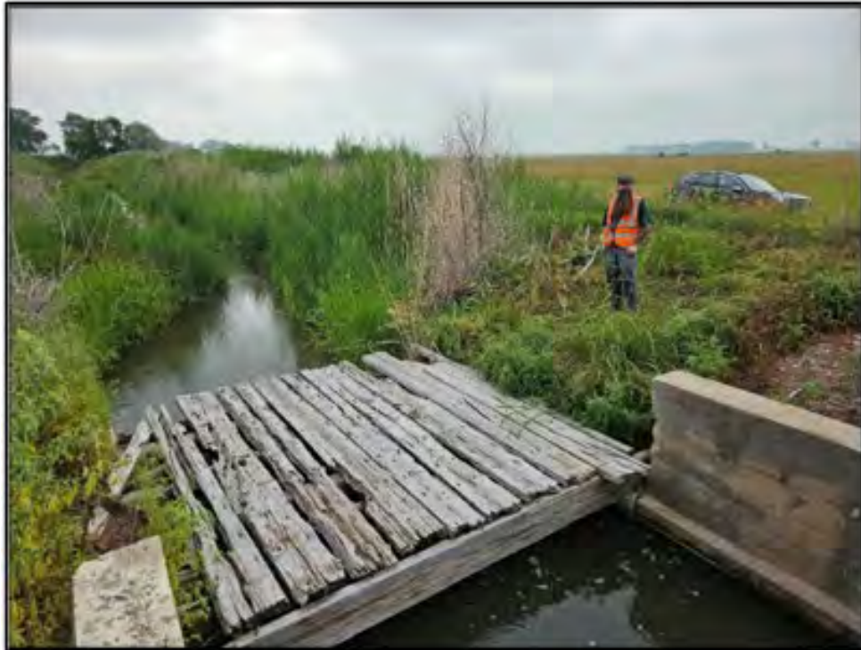
Figure 99. Cody Dillon Canal: Feature 5, decayed wood vehicle bridge. View to the east from the access platform of the headgate (Feature 4). Photograph taken on July 21, 2025.
