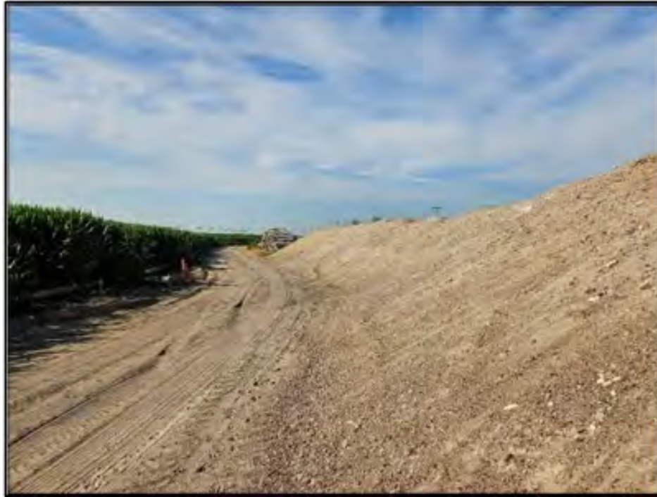
Figure 92. Suburban Canal: Feature 4, sediment and railroad tie stockpile for erosion control. View to the south. Photograph taken on July 19, 2025.
