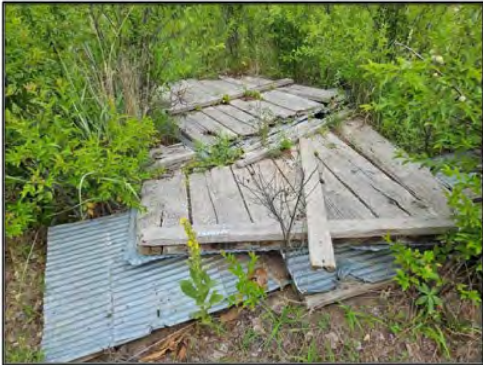
Figure 76. Paxton Hershey Canal: Collapsed remains of old gaging station at Feature 5. View to the east. Photograph taken on July 17, 2025.
