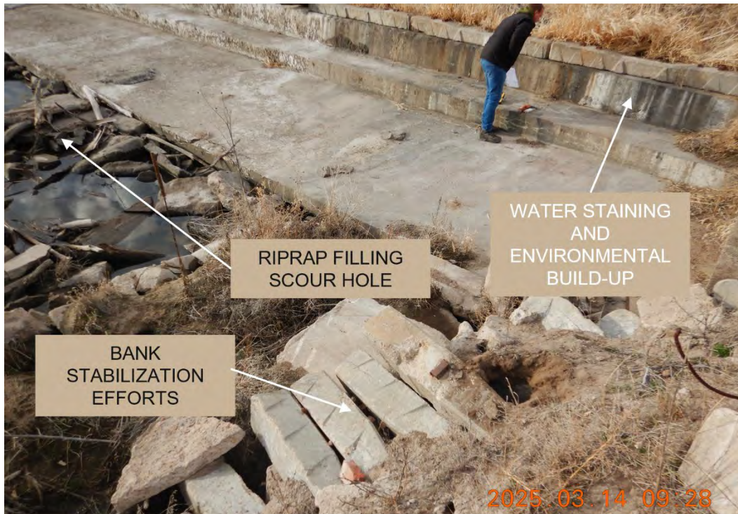
Figure 15. Typical Apron Condition and Environmental Buildup – Downstream End
