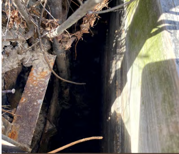
Figure 13. Screw Gate Deterioration
