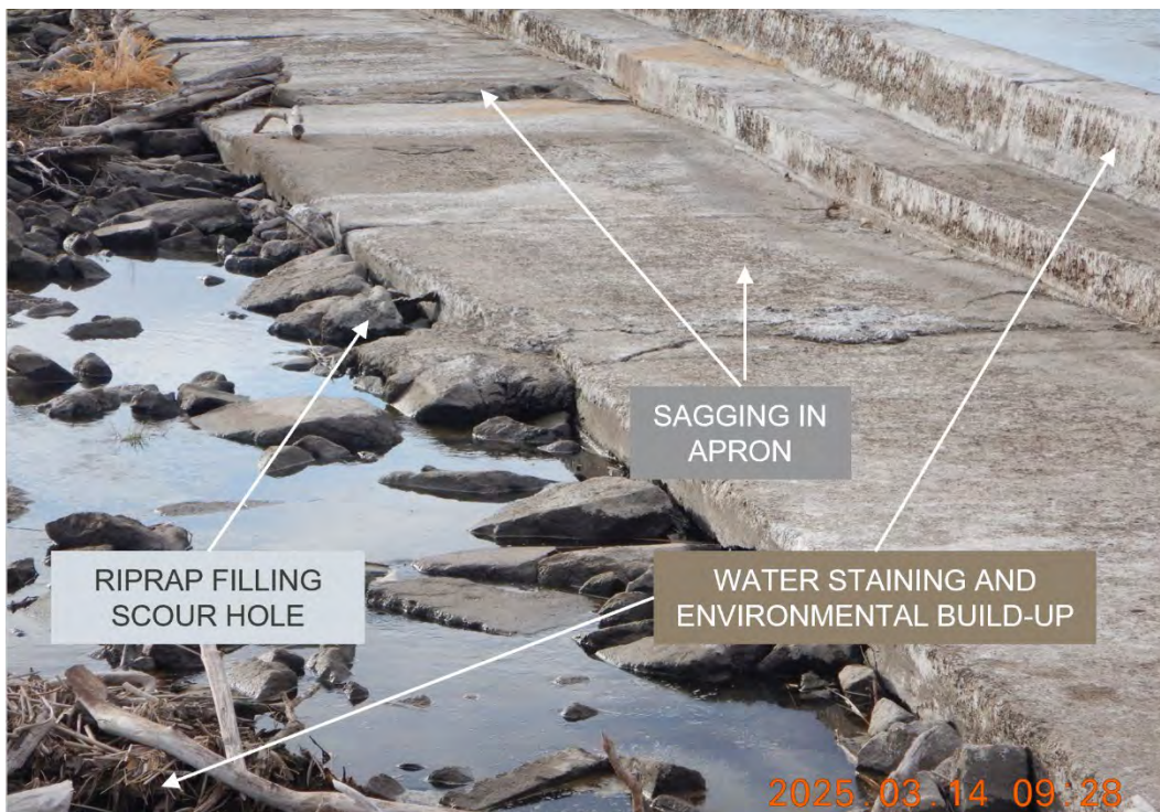
Figure 16. Typical Apron Condition and Environmental Buildup – Downstream End
