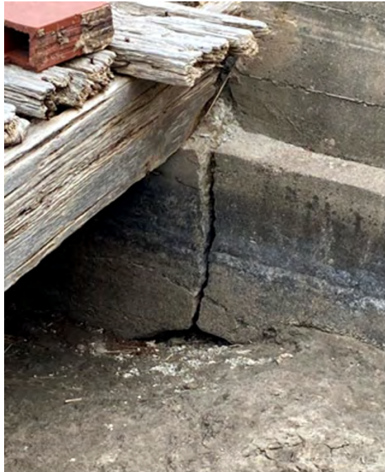
Figure 16. Vertical Crack in Wall Base at Access Bridge.
