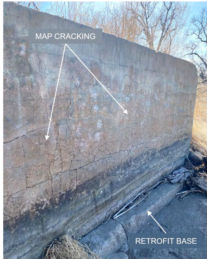
Figure 24. Typical Map Cracking and Spalling
