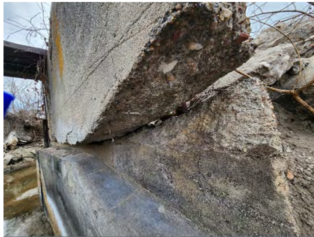
Figure 6. Close-up view of Wall Failure.
