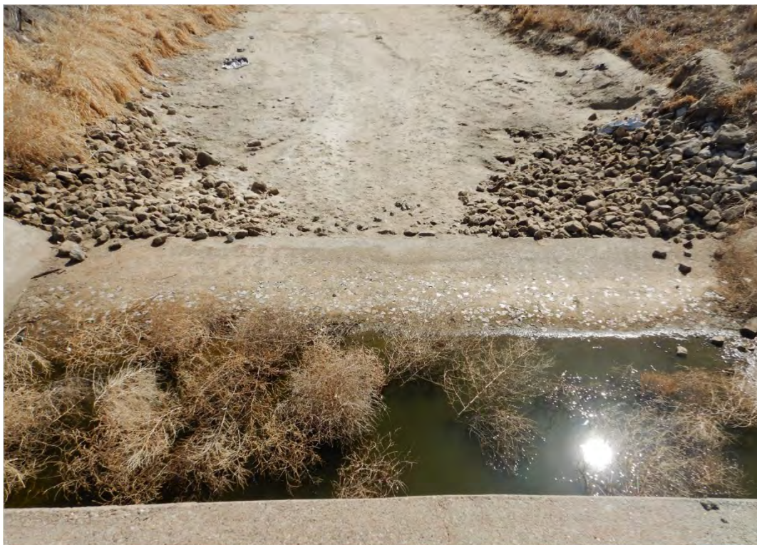
Figure 11. Concrete Apron, Canal Channel Bed, and Ponding Water
