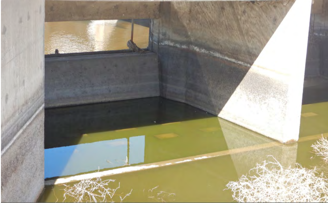
Figure 12. Splash Pad, Baffles and Ponding Water
