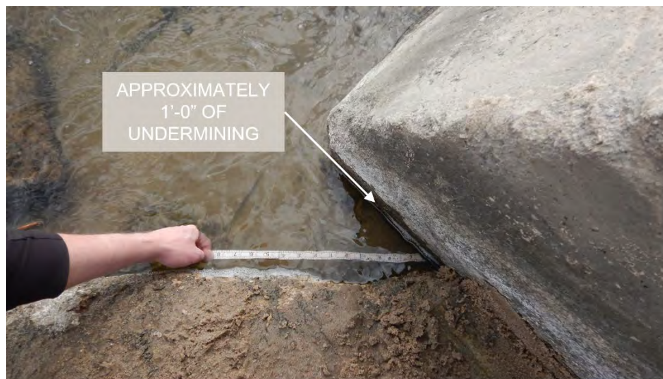
Figure 8. Undermining of North Exterior River Gate Wall
