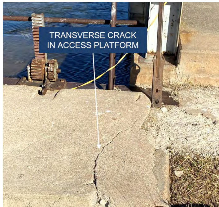
Figure 22. Transverse Crack in Access Platform
