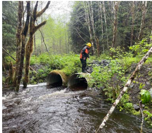
Pictured: Insufficient aquatic habitat for fish due to undersized culverts.
