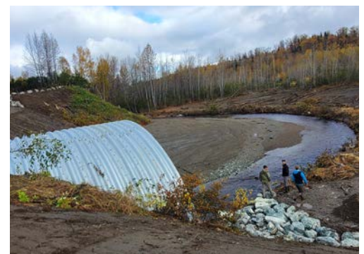
Tyonek TCD is working with many partners including USDA to install fish passage culverts to improve salmon habitat.
