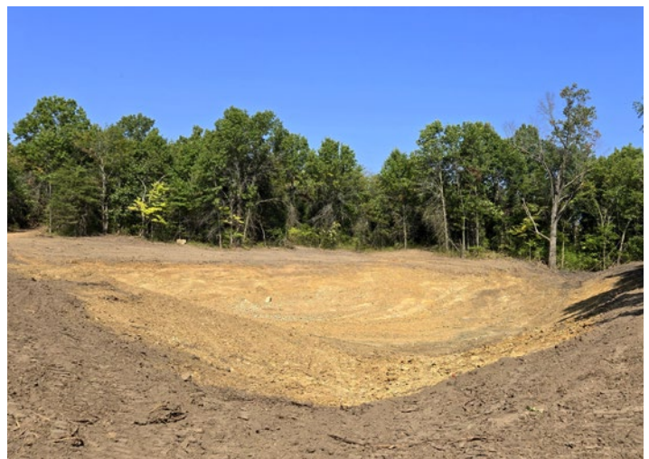
A wide angle of the newly constructed sediment basin on Sept. 11 in the Rathbun Lake Watershed. (Photo by Scott Cagle)
