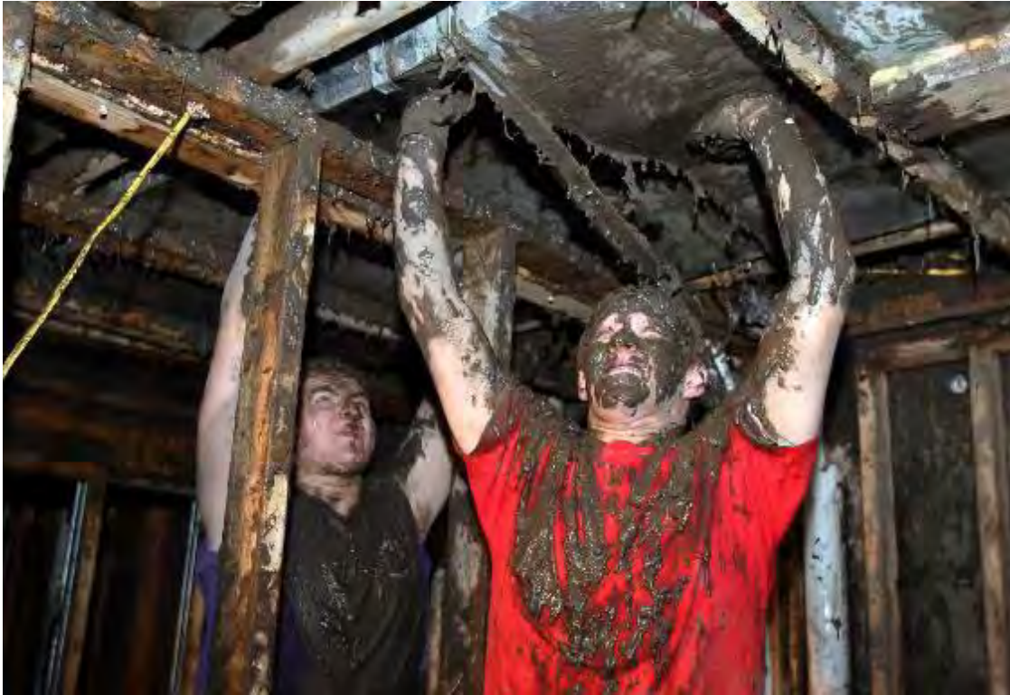
Photo 3. Basement flood damage from September 4, 2012
