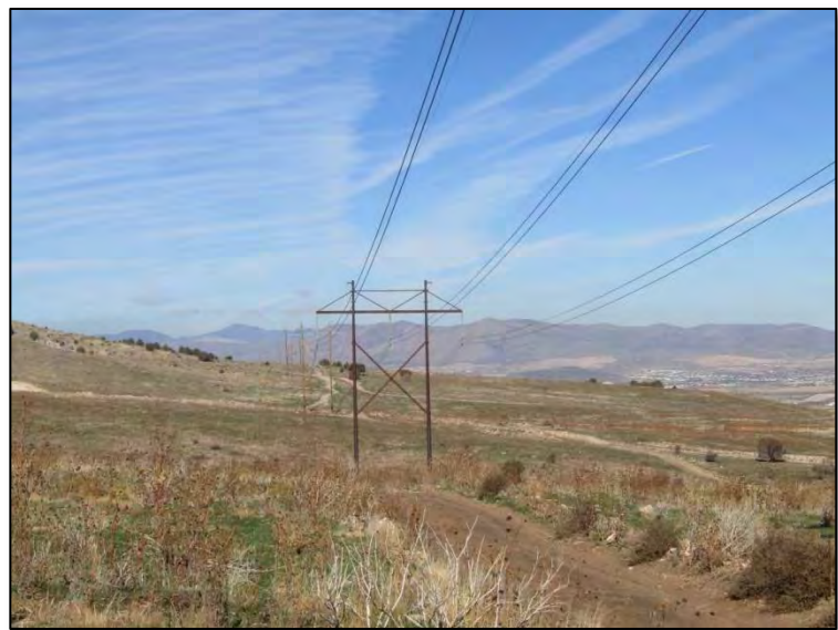
Figure 8. Example of transmission line corridor; looking north
