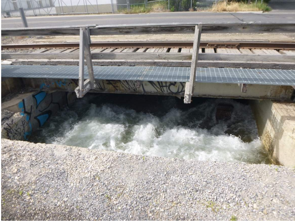
Photo 3. Downstream condition of box culvert at 100 North and 200 East. Note the missing baffle blocks.
