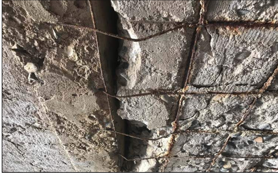
Photo: 200 South Culvert Ceiling Exposed Rebar
