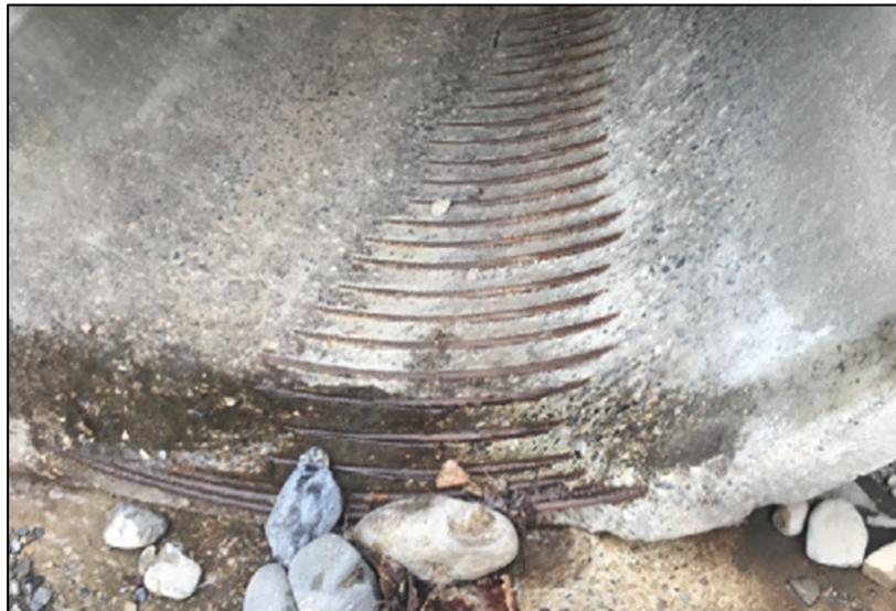
Photo 2. Close View of RCP with Exposed Rebar.
