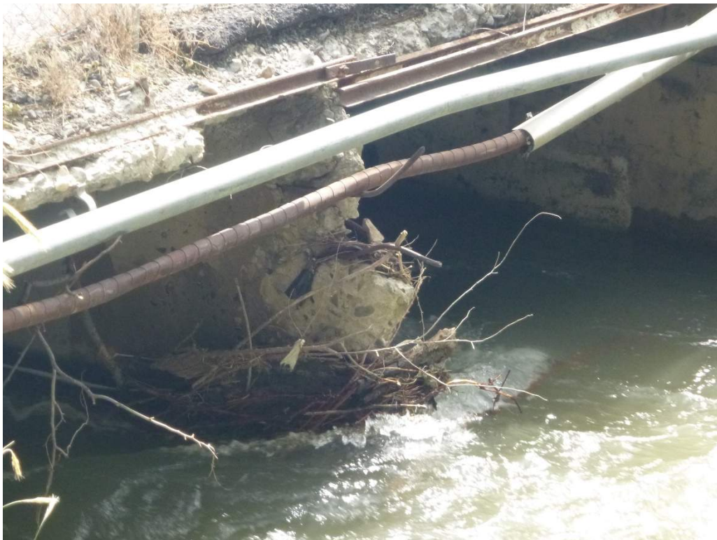
Photo 2. Deteriorating concrete and exposed rebar.
