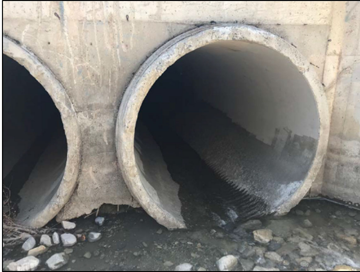
Photo 1. RCP with Exposed Rebar.
