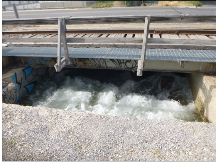
Photo 9. Downstream Condition of Box Culvert at 100 North and 200 East. Note the missing baffle blocks.
