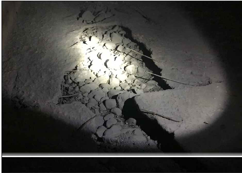
Photo: Box Culvert Floor Erosion
