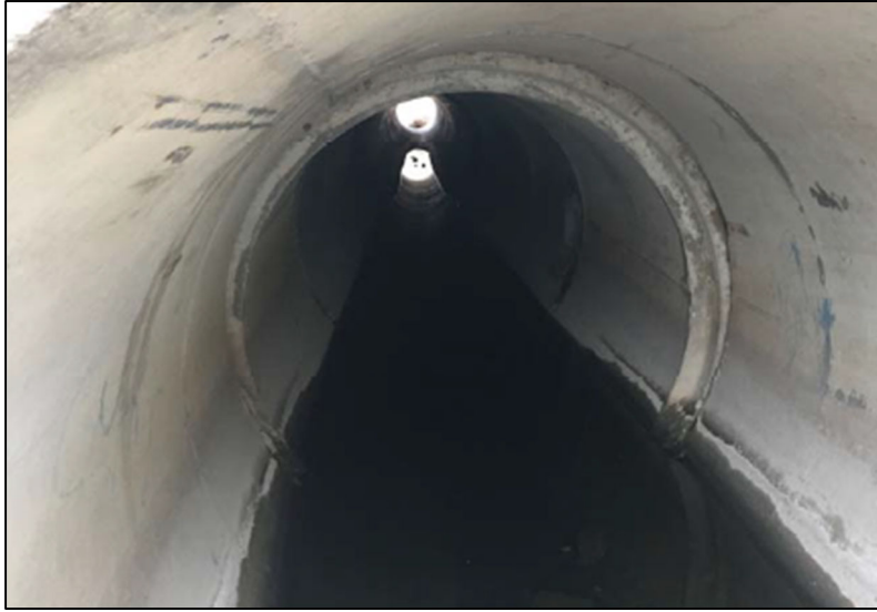
Photo 3. RCP with Wide Gaps at Joints.
