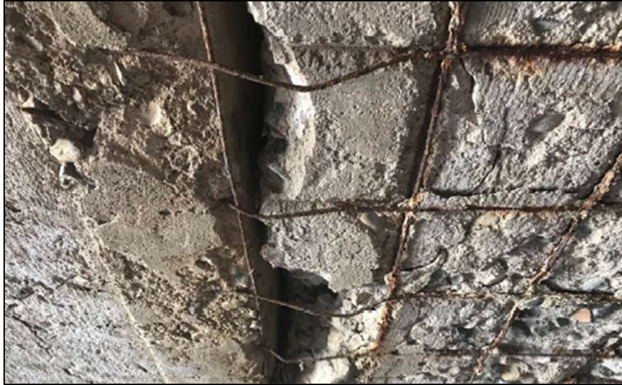
Photo 14. 200 South Culvert Ceiling Exposed Rebar.
