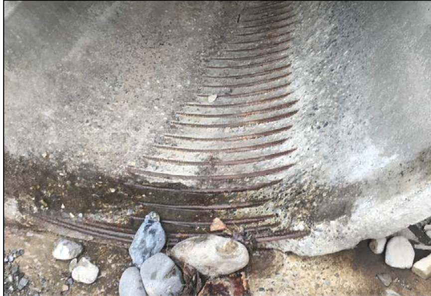
Photo: Close View of RCP with Exposed Rebar
