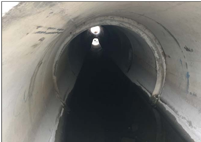
Photo: RCP with Wide Gaps at Joints
