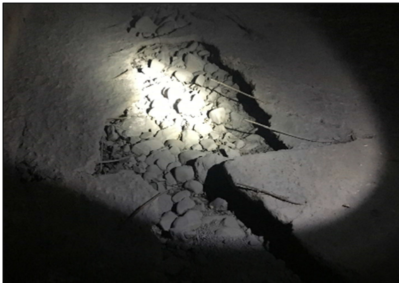
Photo 10. Box Culvert Floor Erosion.
