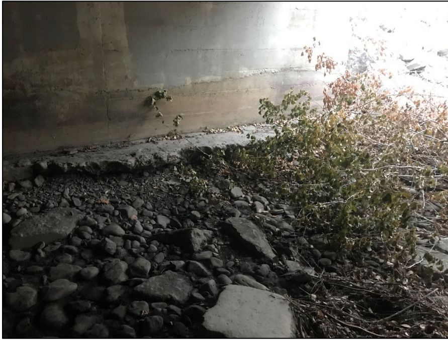
Photo 5. Missing Floor and Undercutting of Walls.
