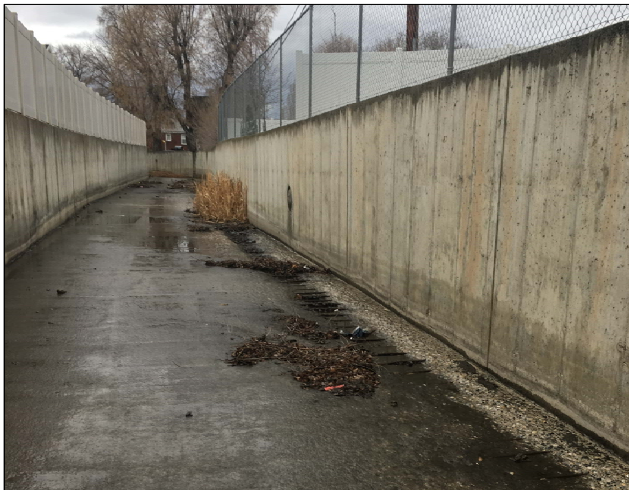
Photo: Open Channel Floor Rebar Exposed
