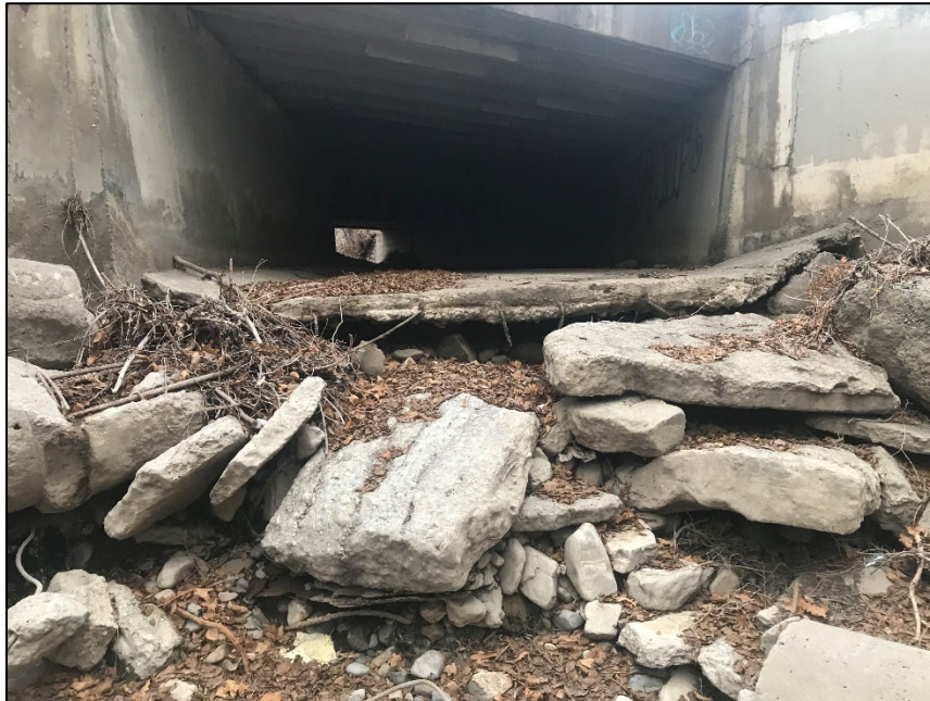
Photo 6. Downstream Undercutting and Missing Apron.
