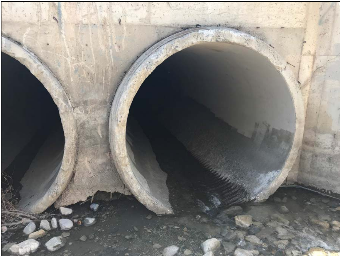
Photo: RCP with Exposed Rebar
