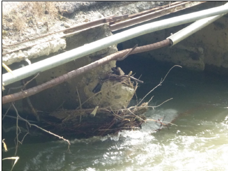
Photo 8. Deteriorating Concrete and Exposed Rebar.
