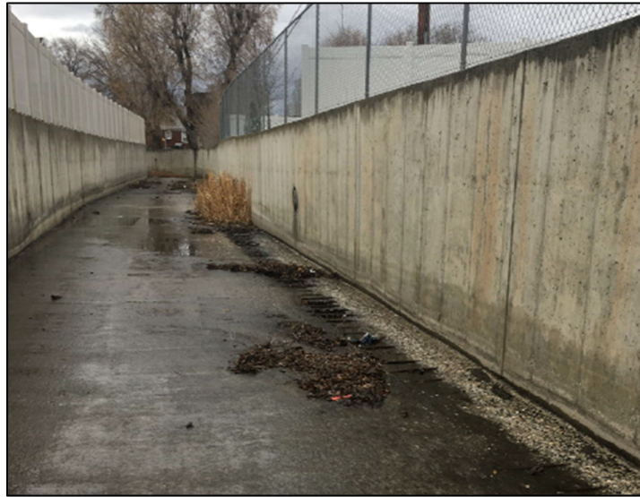
Photo 11. Open Channel Floor Rebar Exposed.
