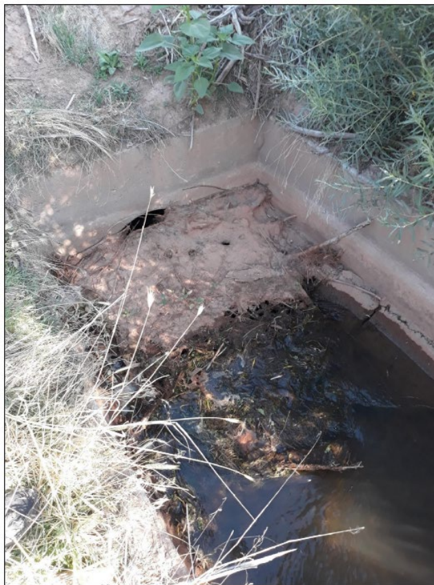
Figure 3-13: South & West Field Double Ditch Pipe Inlet Covered in Sediment and Debris
