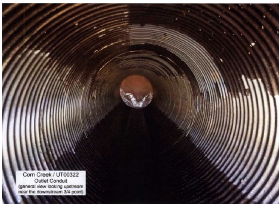
Figure 3-8: 60-inch Conduit (DWRi 2019)
