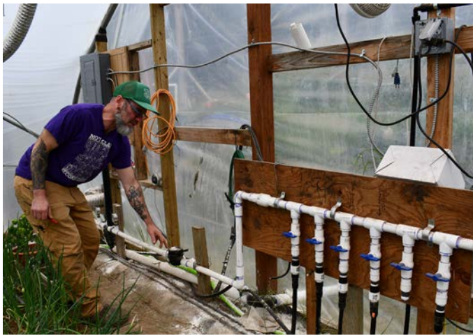
NRCS can help producers install irrigation systems to improve water use efficiency for producers growing crops inside of a seasonal high tunnel.
