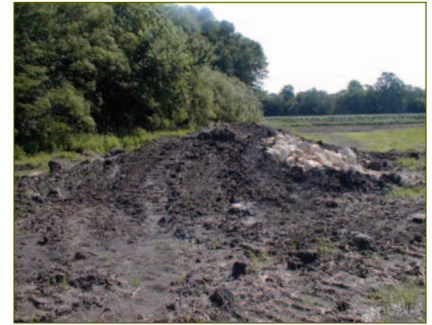
Newly constructed snake hibernacula on a Wetland Reserve Program easement in Clinton County, Iowa.
