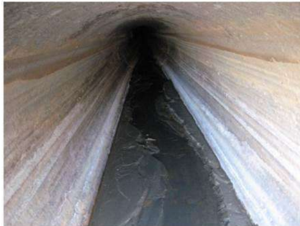
Photo 15: Interior of outlet pipe showing sediment accumulation. (12/11/2014)
