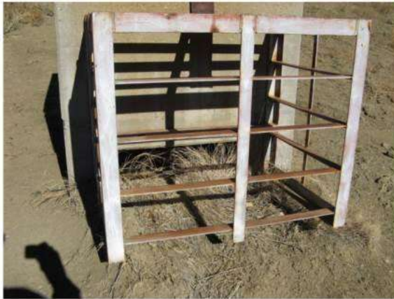
Photo 9: Principal spillway riser inlet showing vegetation at inlet opening. (12/11/2014)
