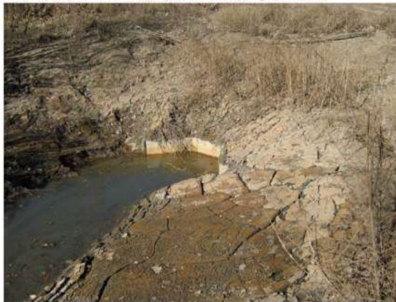
Photo 10: Low level inlet showing sediment accumulation and water impounding at inlet due to deteriorated and corroded low level inlet pipe downstream of the concrete inlet. (12/11/2014)
