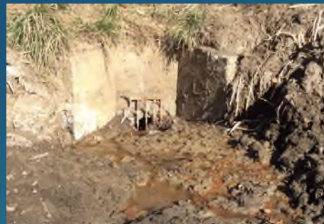
Low-Level Drawdown Pipe Inlet
