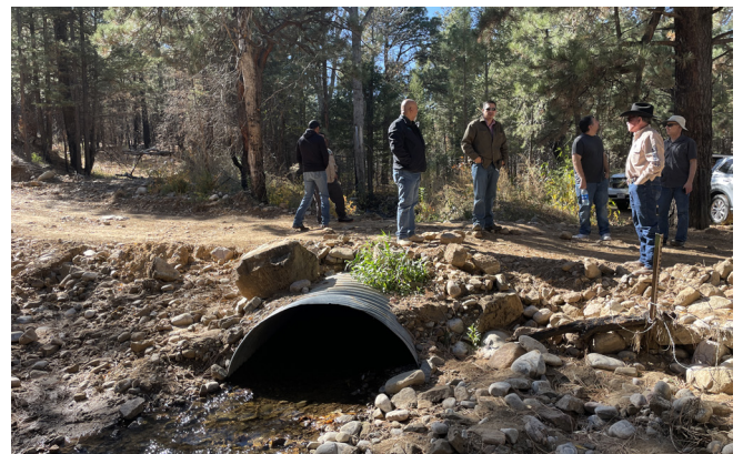
NRCS NM assesses a damaged Acequia.
