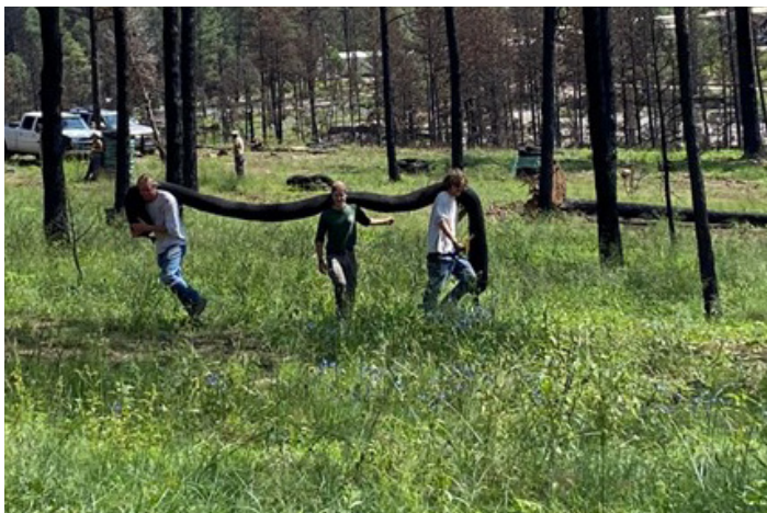
EcoServants, a local non-profit organization made up of high school and college students assist NRCS in laying out wattles.
