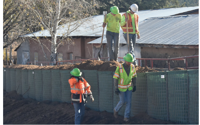
Local contractors installing point protection bags to protect homes from potential flooding.
