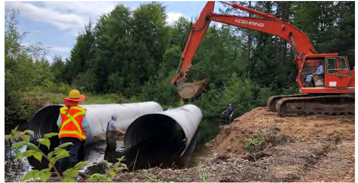
Two 87" x 63" x 50' aluminized steel arched culverts being placed in the stream bed. Mary King oversaw the construction.
