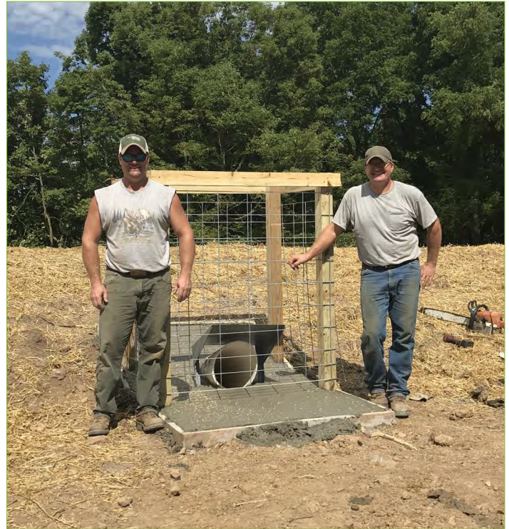
Chris Hammell (left) and Eric Hammell (right) by a dam they constructed.
