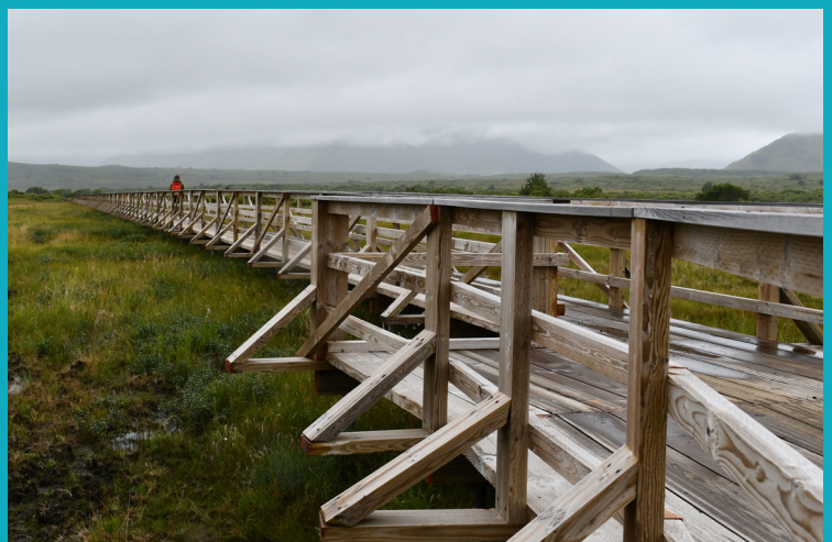
The helical pile boardwalk has side safety railing and several turnouts for ATVs or UTVs.
