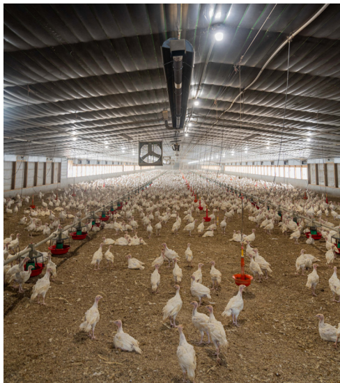
John Baker raises about 28,000 turkeys at a time across three barns on his farm in Salem, Indiana. He has worked with NRCS to implement multiple energy efficiency practices including an energy audit, LED lighting, attic insulation and heaters. Photo Credit: Brandon O'Connor.
