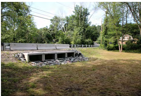
The roadway was raised to allow safe access and a box culvert was installed to allow storm water to flow under the road and back to the Pocasset River. (AFTER)
