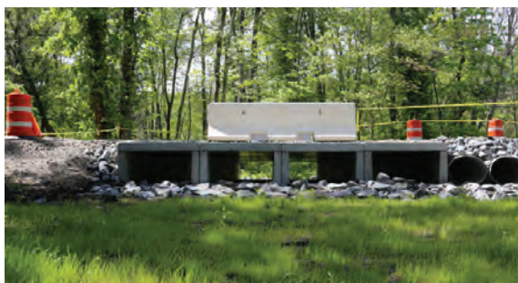
A box culvert was installed to allow storm water to flow under the road and back to the Pocasset River.
