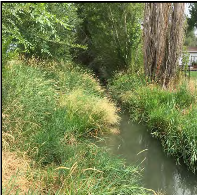
Representative conditions along Ashley Canal segment surveyed.
