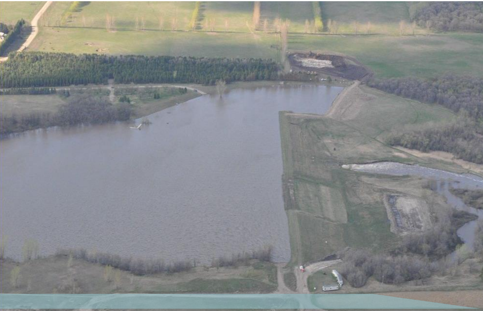
Renwick Dam in Pembina County, ND – May 2013. Photo Courtesy of Civil Air Patrol
