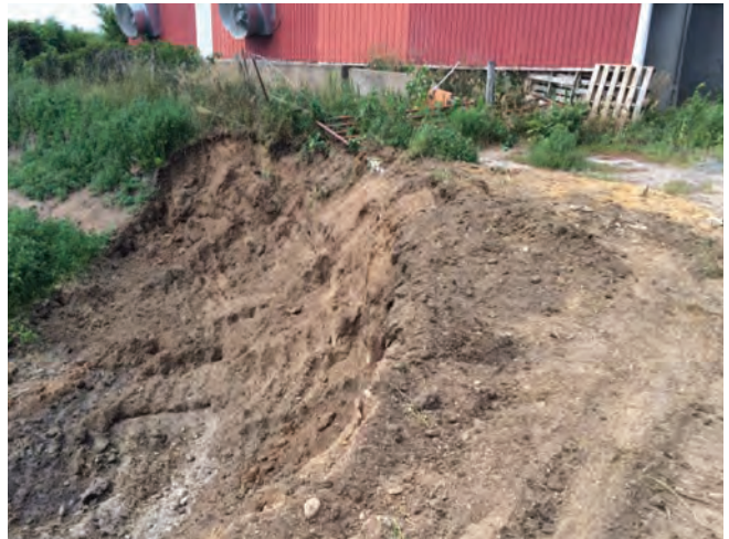
Wall cleaning to remove all the manure/soil mix to allow for clean fill to reclaim the pit area.
