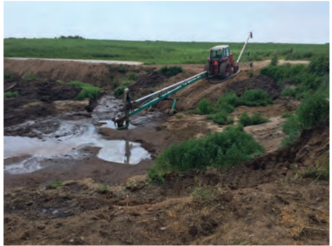
Emptying the pit for the last time. This is done to remove as much manure and water as possible prior to the abandonment process.
