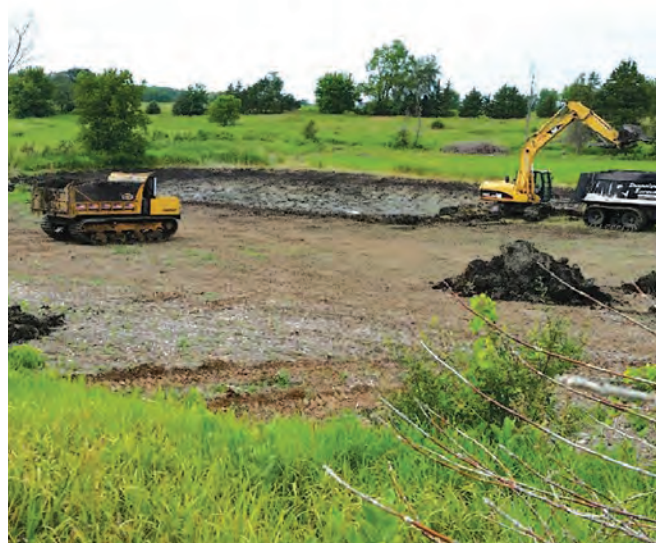
A pond is dug in a lowland area of the Raasch property during easement restoration construction.
