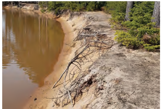
Project site prior to restoration. Note the tree root and erosion issues.
