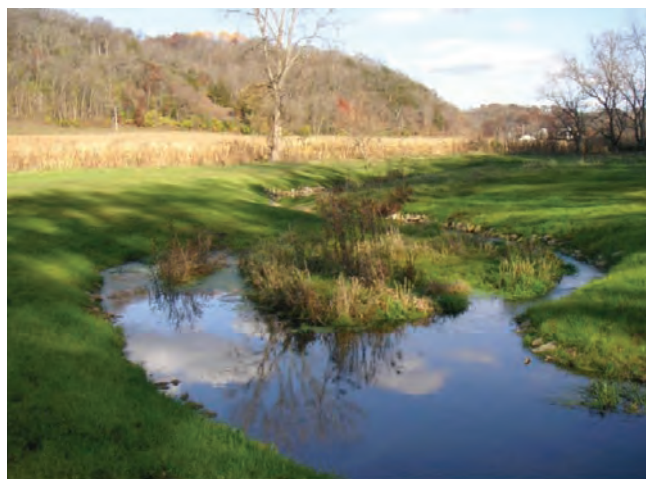
After construction. Banks were shaped, riprap put into place, then top soil was spread on the banks and they were seeded down. Also, you can see where a backwater refuge was constructed.
