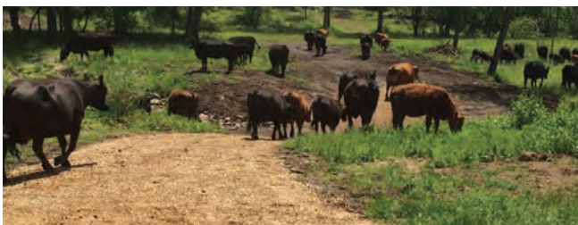
During (top) and after (bottom) streambank repair and the installation of rip rap and a ford stream crossing and seeding.
