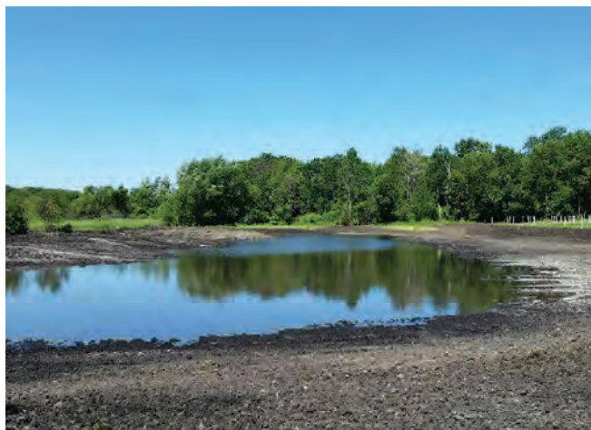
A newly created shallow scrape is thriving and filled with water after construction in a lowland area on the property.
