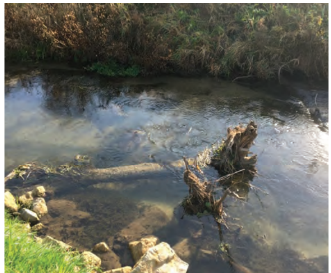
Spring Coulee Creek after streambank protection and fish habitat installation. Lunker structures, instream wood placement and instream rock placement provide habitat for trout.
