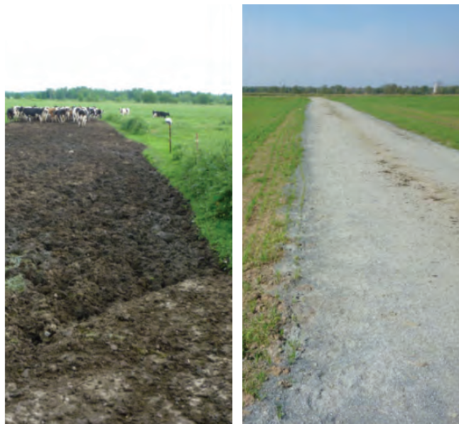
(L) The Bolstad lane for cattle traffic before technical assistance. (R) The lane after design and construction.
