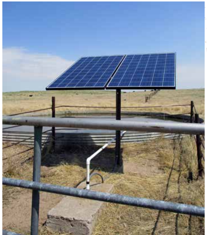
Solar livestock watering system to help facilitate grazing management in a remote area.
