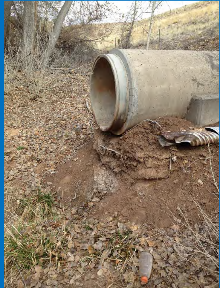
Principal Spillway Outlet Pipe, Toe Drain and Undercutting at Outlet Pond
