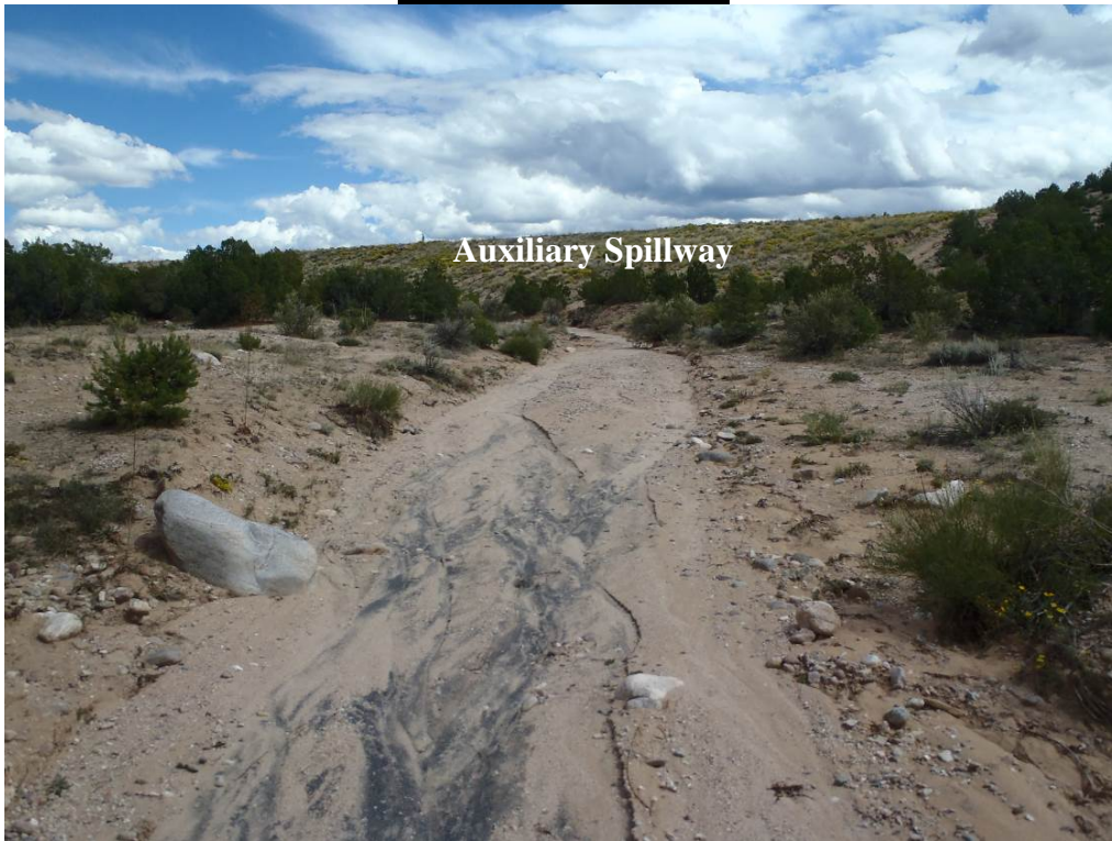
Photograph 9 (9/14/16) – Looking upstream along the Cañada de Ojito with the auxiliary spillway in the background.
