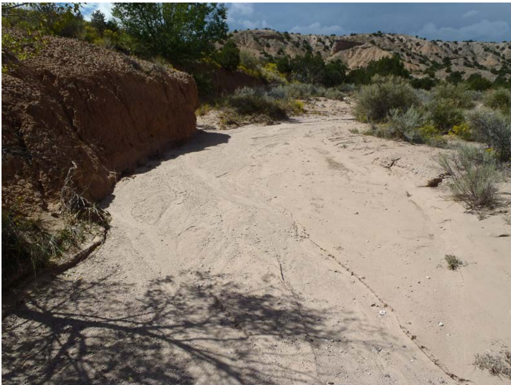
Photograph 13 (9/14/16) – Looking upstream along the redirected Cañada de Ojito adjoining the toe of the diversion dike.
