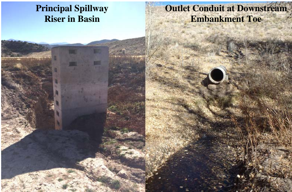
Photograph 4 (12/13/17) – Looking at the principal spillway riser and outlet conduit of the dam.
