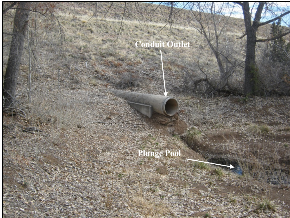
Figure 1-5. Principal Spillway Conduit Outlet (View of principal spillway conduit discharge point and plunge pool)
