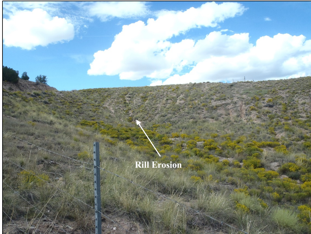
Figure 1-3. Embankment Groin Rill Erosion (Looking at rill erosion on one of the downstream embankment groins)
