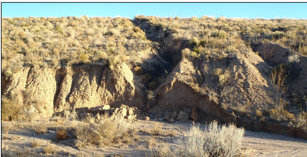
Figure 1-8. Auxiliary Spillway Rill Erosion (Standing in the Cañada de Ojito drainage looking southeast at auxiliary spillway exit slope erosion)
