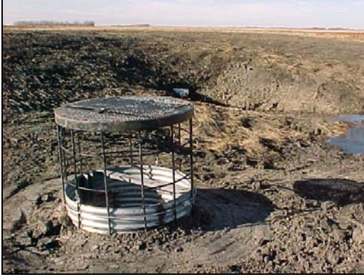
A water control structure installed on a large drained semi-permanent wetland along the Red River in Walsh County
