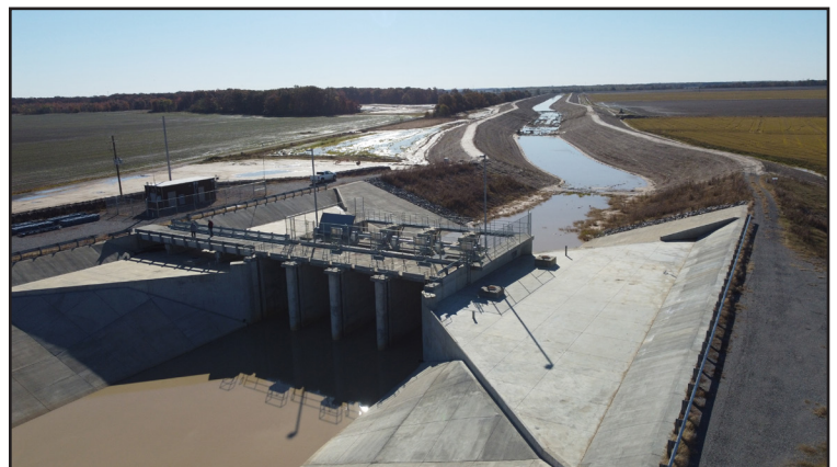
Canal 1000 starts below the regulating reservoir outlet structure in the foreground. NRCS and the WRID are constructing the canal.
