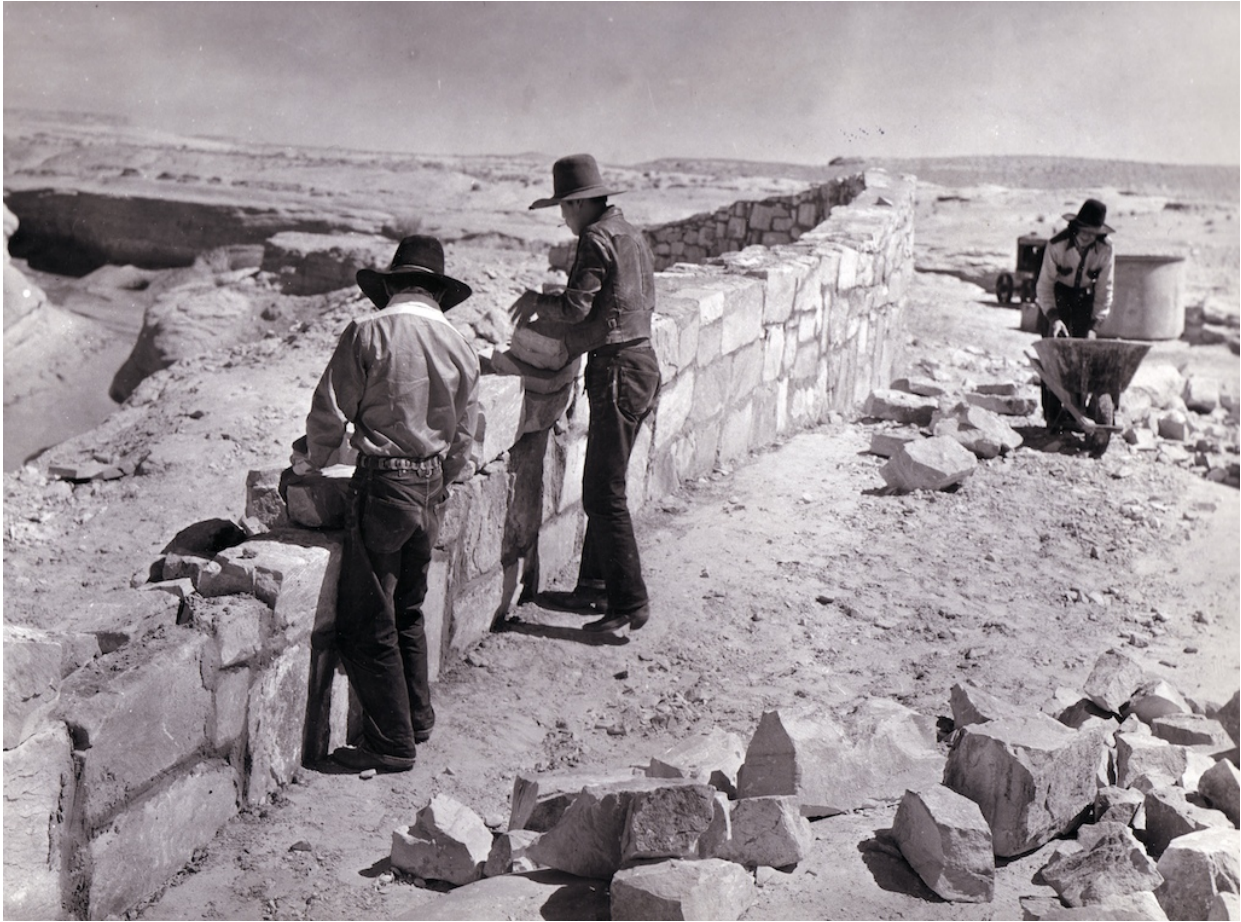
Navajo CCC workers build a diversion. Tuba City, Arizona (75N-Nav-296 National Archives and Records Administration, College Park, Maryland)
