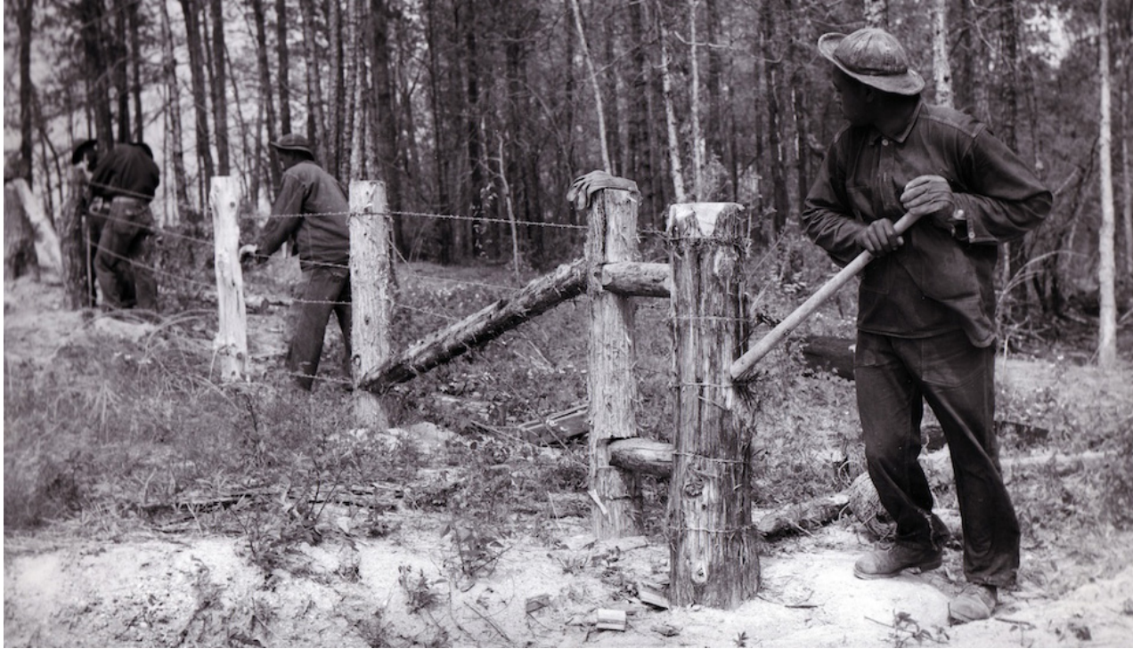
CCC enrollees building fences. Camp SCS-NC-5, Yanceyville, North Carolina. 35G No.287 (National Archives and Records Administration, College Park, Maryland)
