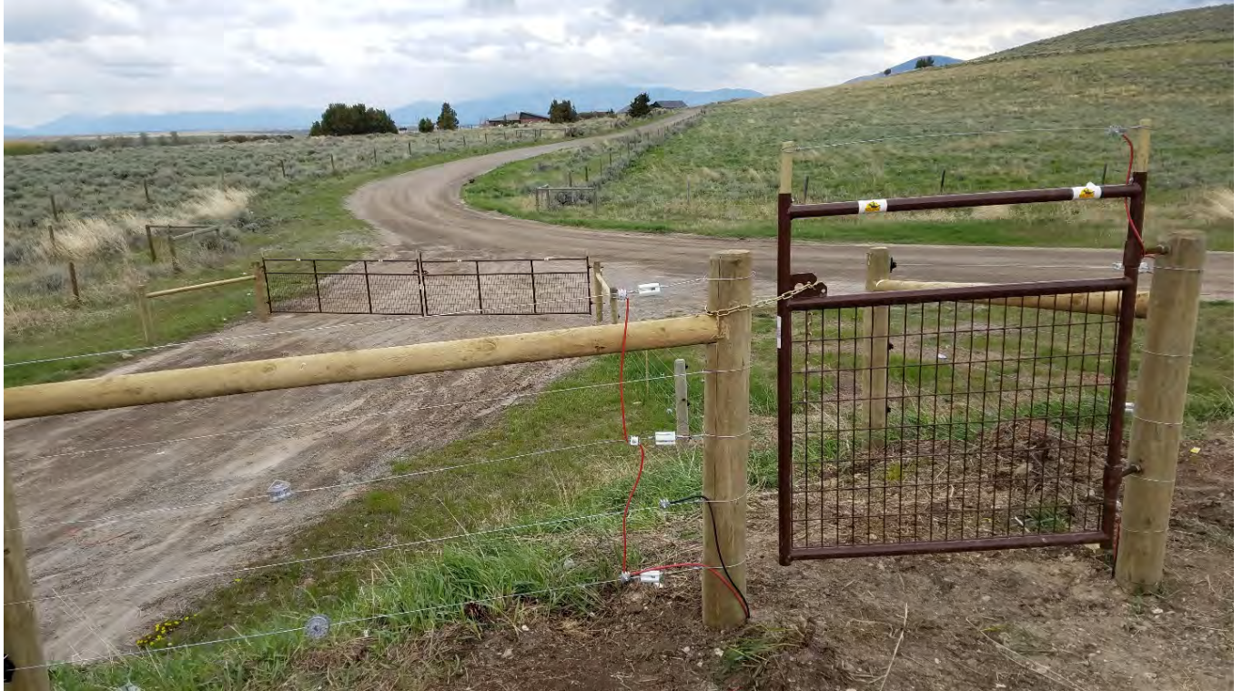
Figure 4. Electric Fence installed to deter grizzly bears from entering a ranch headquarters area. This installation uses an electric wire over top of gates to prevent climbing.
