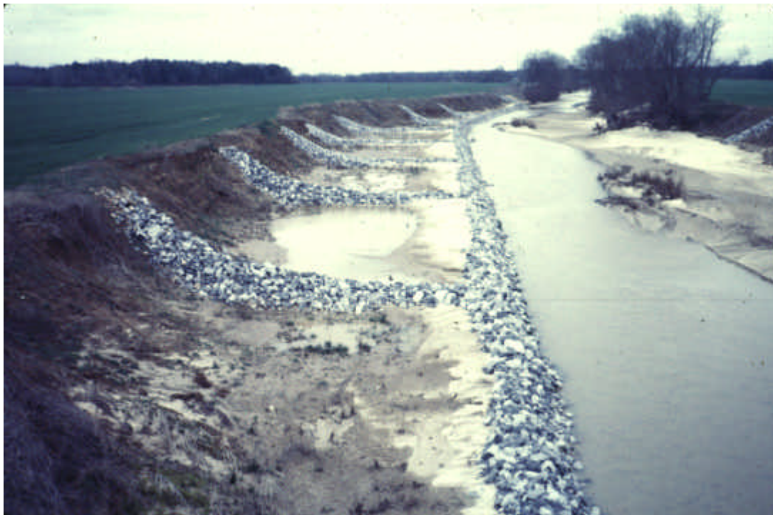
Figure 7.11 Longitudinal Stone Fill Toe Protection Riverward of High Bank With Tiebacks
