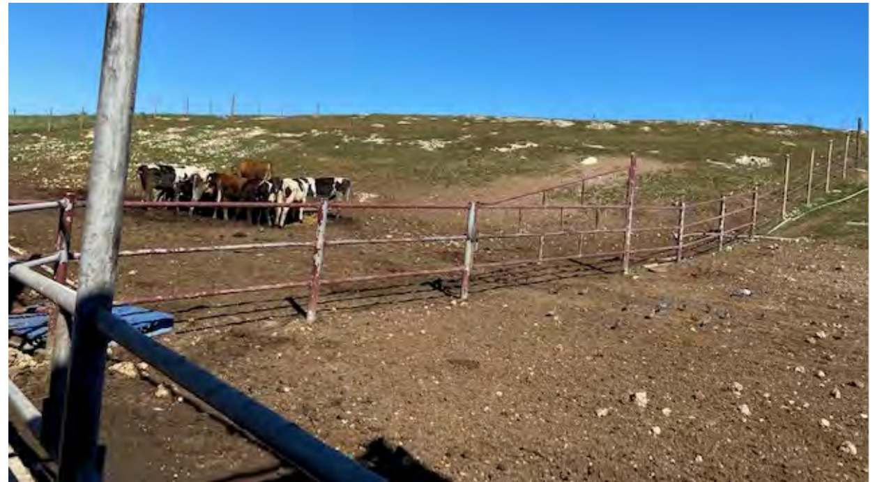
Figure 34. Picture after 1 year of HUAP implementation. Performing well. Drainage is Really Important
