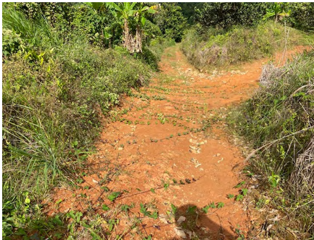
Figure 2: Steep farm road highly eroded. Jayuya, PR
