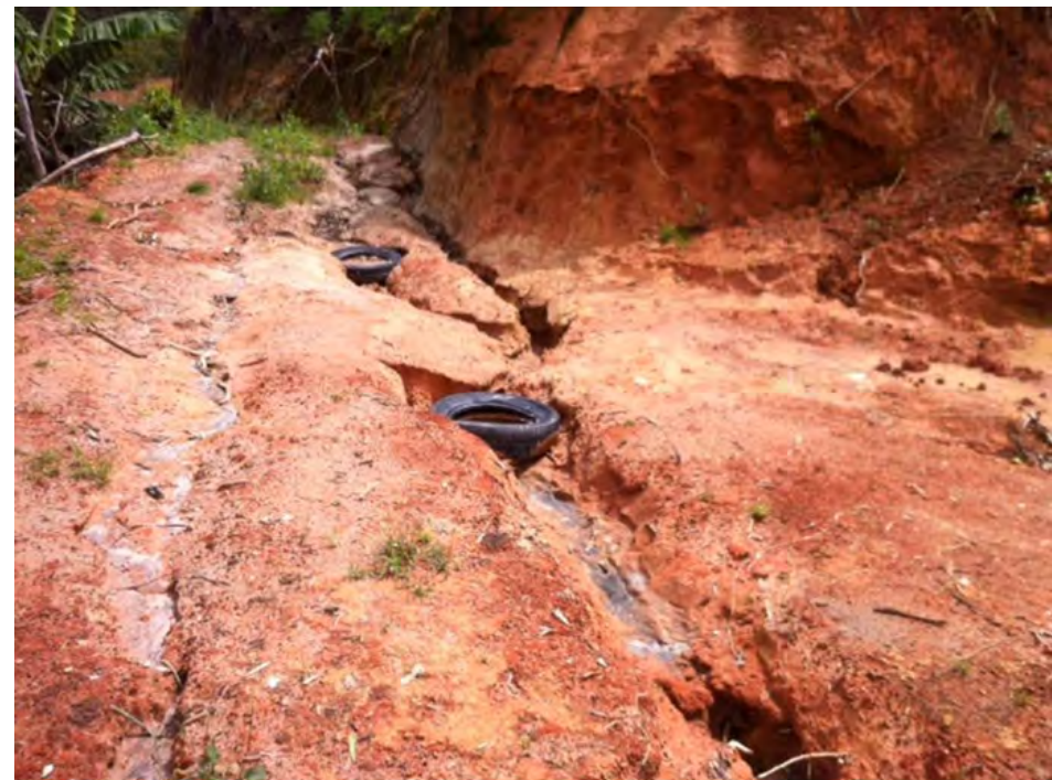
Figure 1: Farm road highly eroded. Jayuya, PR
