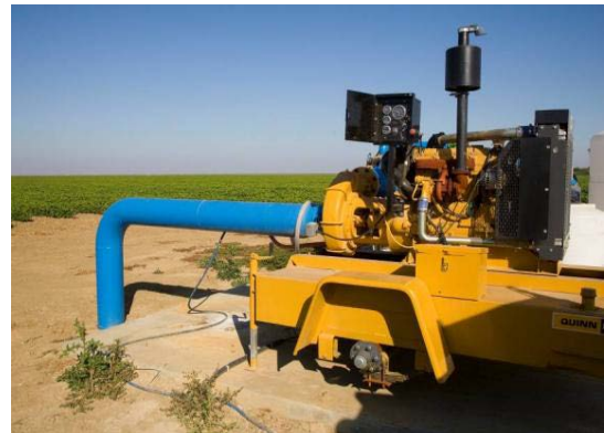
Figure 6.6 Irrigation system pump.
