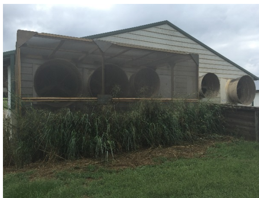
Figure 2.10 An experimental windbreak wall installed at a swine house exhaust fan.
