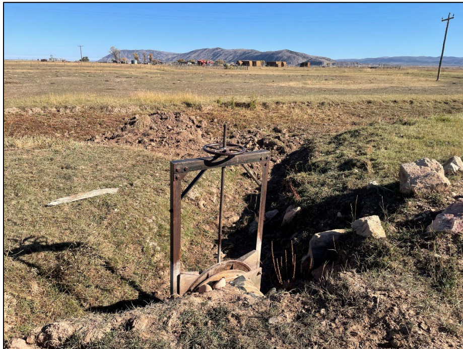
Photo 11: The Shulthess Diversion on Woodruff Creek lies in a heavily grazed pasture. The canal adjacent to this diversion is dry.
