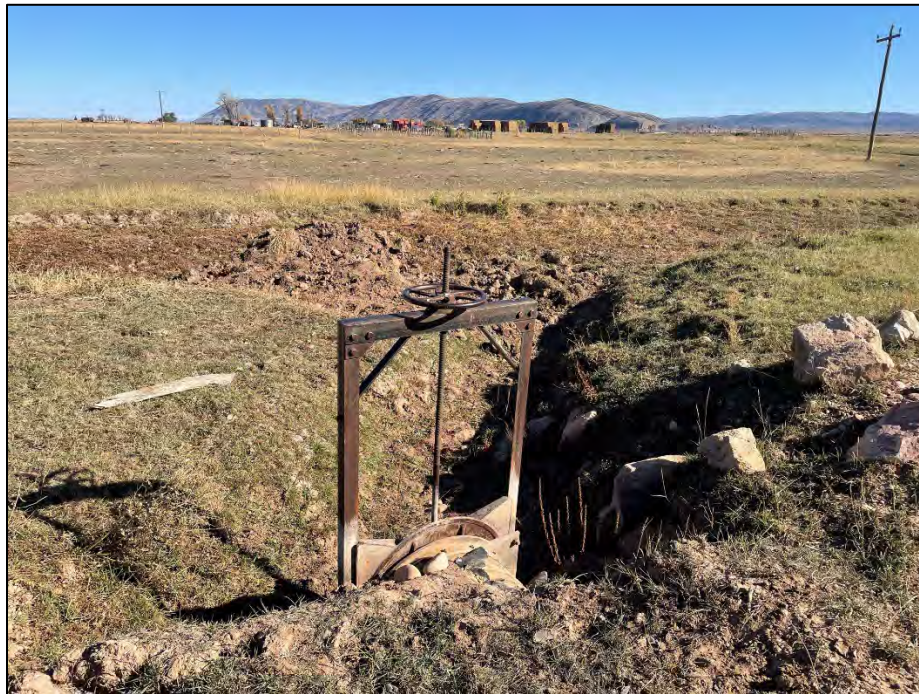
Photo 11: The Shulthess Diversion on Woodruff Creek lies in a heavily grazed pasture. The canal adjacent to this diversion is dry and the edges are eroded.
