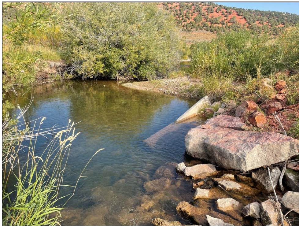
Photo 4: Birch Creek downstream at the Putnam/Cornia Diversion. Riprap and concrete have been placed in the creek.
