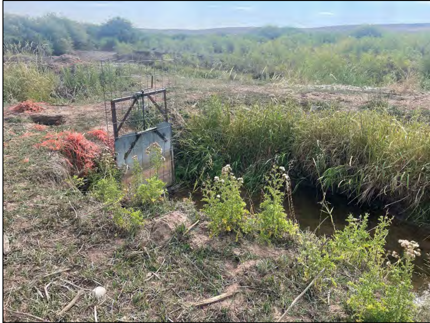
Photo 6: Frazier #1 Diversion on Woodruff Creek. Baling twine debris and dense grasses are present around and in the diversion.
