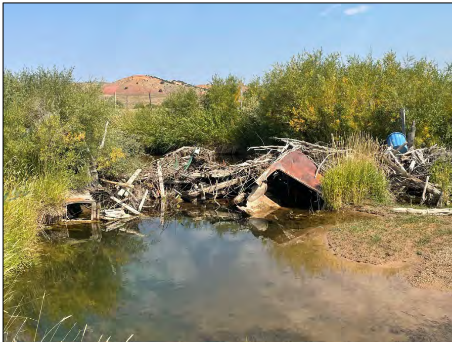
Photo 7: Eastman Diversion #2 on Woodruff Creek. Old vehicles and human made debris are within the diversion structure.
