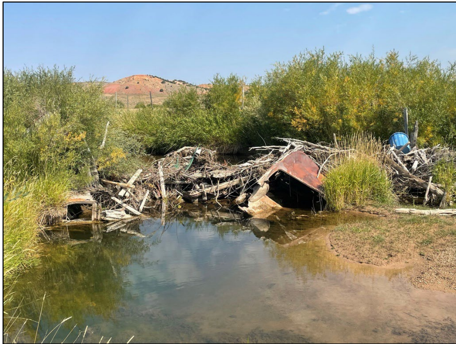
Photo 8: Eastman Diversion #2 on Woodruff Creek. Old vehicles and human made debris are within the diversion structure.
