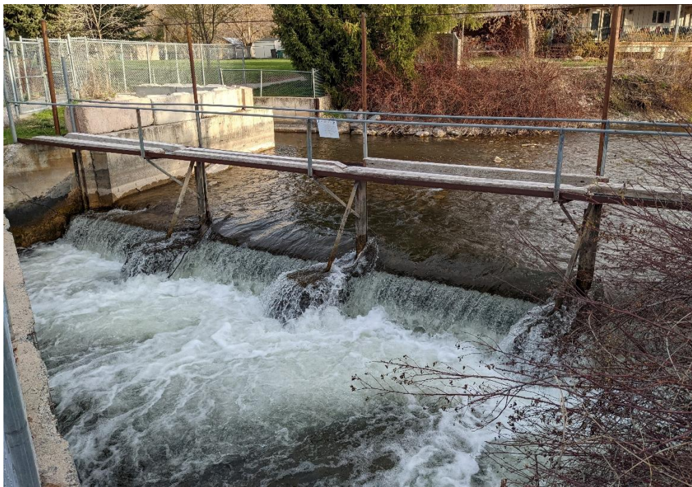
Figure 2-1. Existing Crockett Diversion with approximately 120 cubic feet per second (cfs) of water
