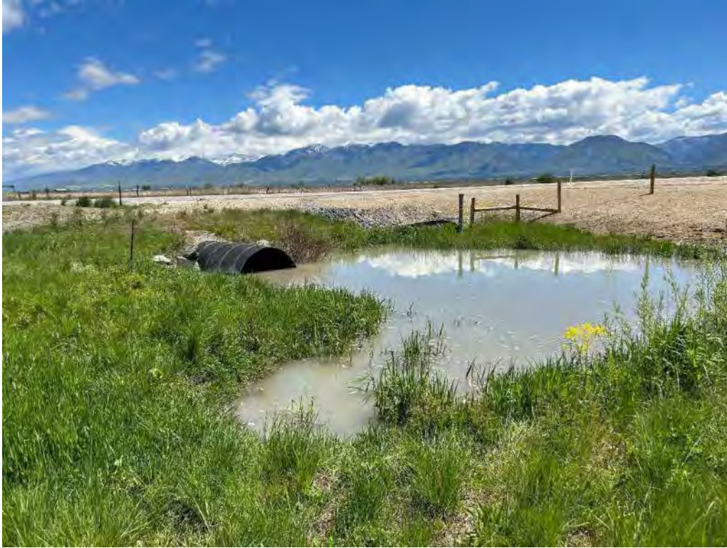
Photograph 13: Northeastern view of canal 4 discharging to Logan River, culvert, and road prism.
