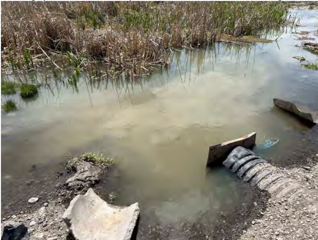
Photograph 19: West view of blocked culvert on ditch 38 and associated flooding.
