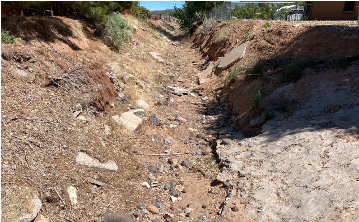
Photograph C-17. Damaged drainage channel in Diamond Valley.
