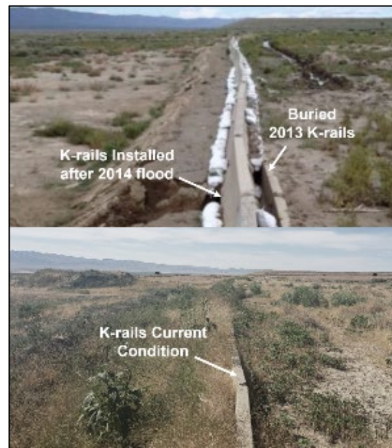
Figure 2-2. 2014 K-Rails and Current Condition
