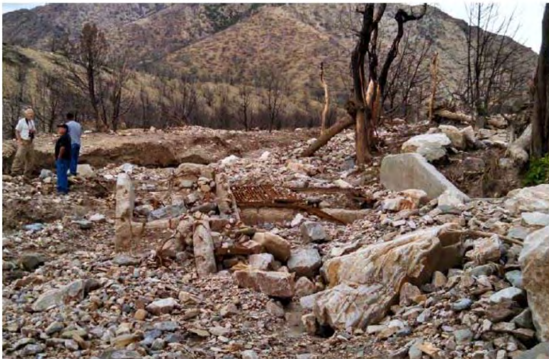
Photo 2. Washed out diversion structure following the 2014 event. (USACE 2018 Figure 10)
