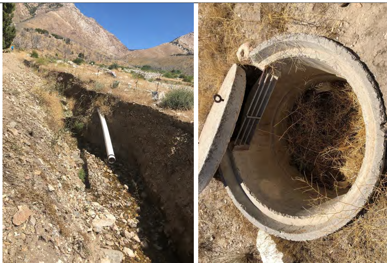
Figure 24. Destroyed Pipeline and Manhole Example 2
