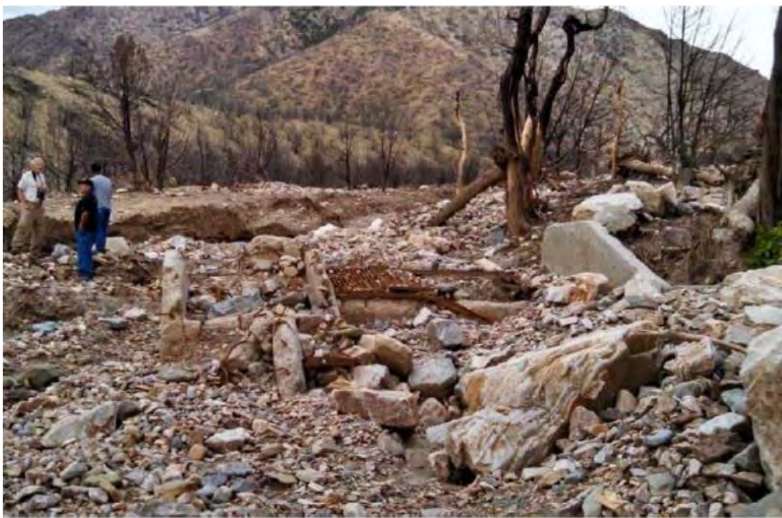
Figure 8. Water Intake structure destroyed in Indian Hickman Canyon
