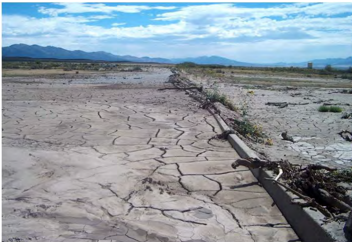
Figure 9. Sediment and debris accumulation upstream of K-rails installed in 2013
