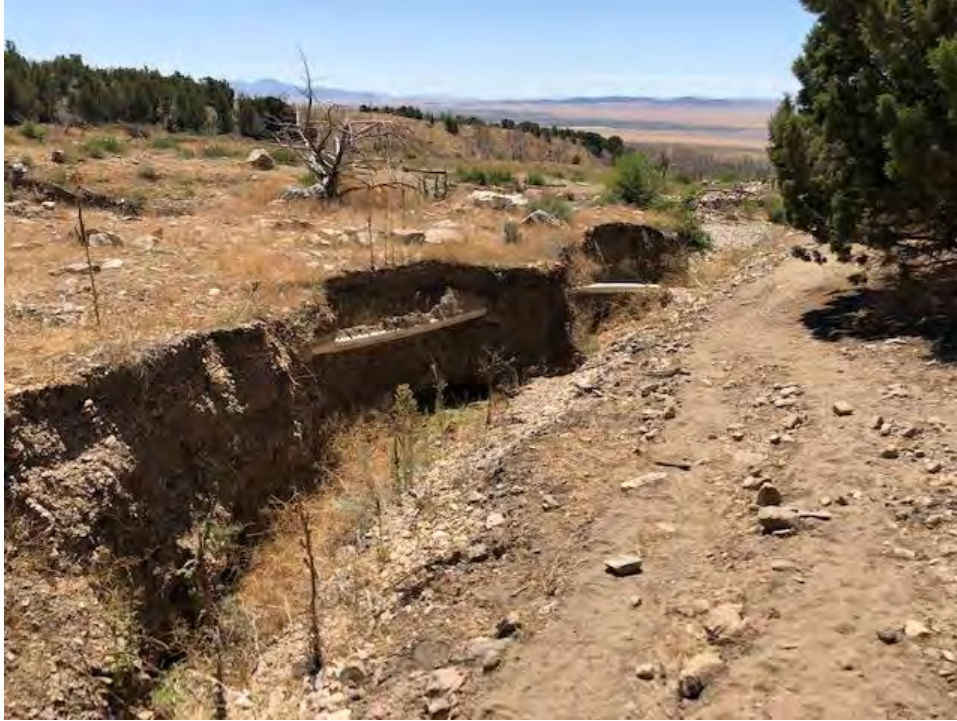
Photo 3. Washed-out pipeline in August 2019.
