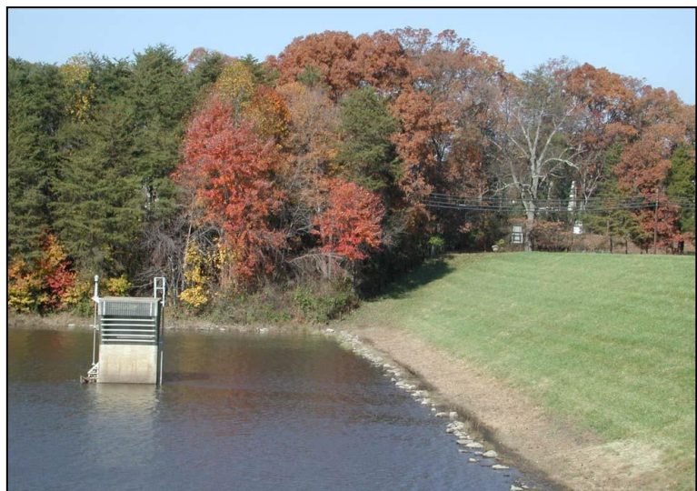
Pohick Site 2, known as Lake Barton, protects homes, businesses, four major roads and several railroad bridges from flooding.
