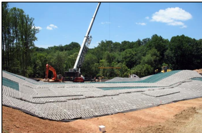
Articulated concrete blocks are installed to provide erosion control on the auxiliary spillway at Woodglen Lake.
