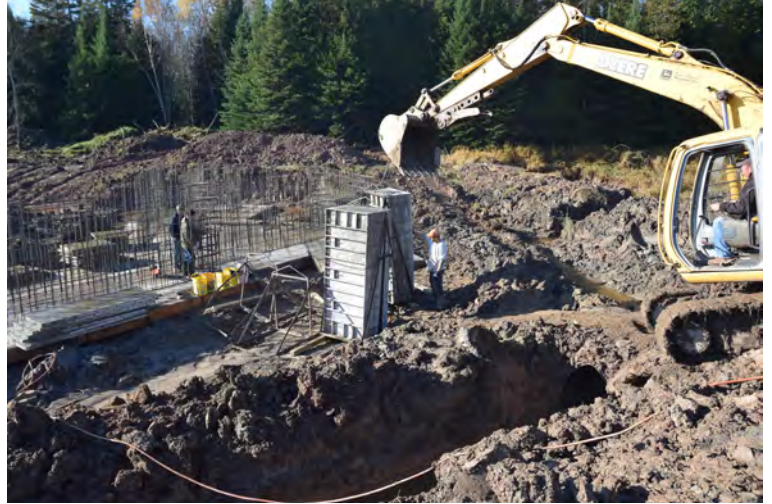
Workers were busy constructing a stream habitat improvement and minnow barrier for the Sault Ste. Marie Tribe of Chippewa Indians in early November (above). The project will be completed in 2017.
