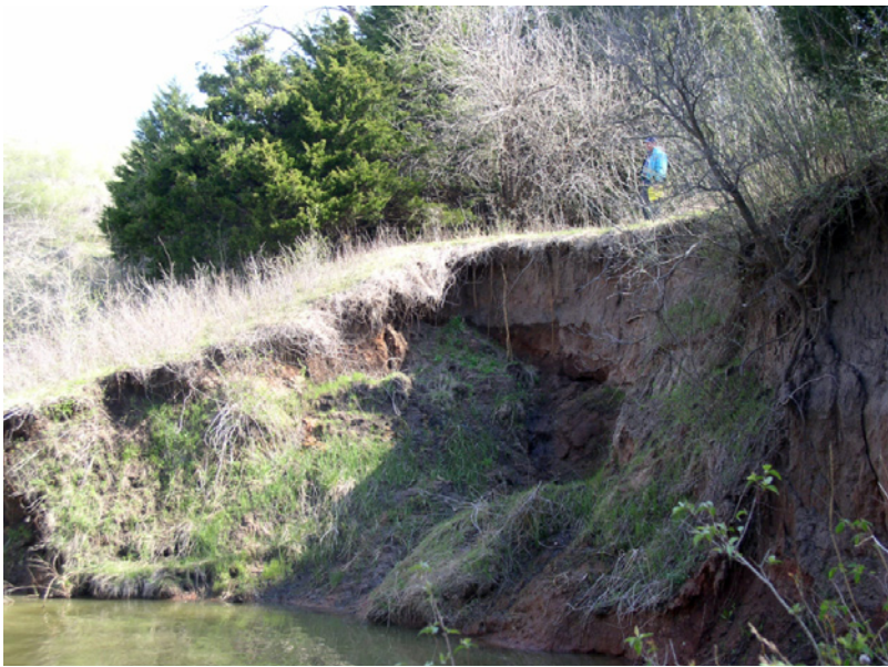
An inspector assesses the severity of the erosion on the backslope of the dam.
