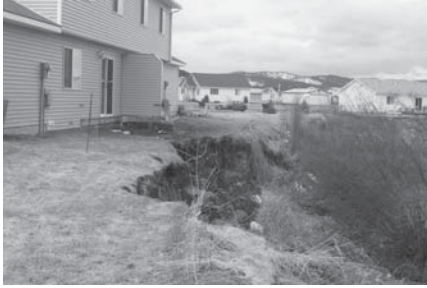
Photograph of a landslide by Mary McDonald Pochelon, Soil Conservation Technician, USDA, NRCS, Kalispell, Montana.
