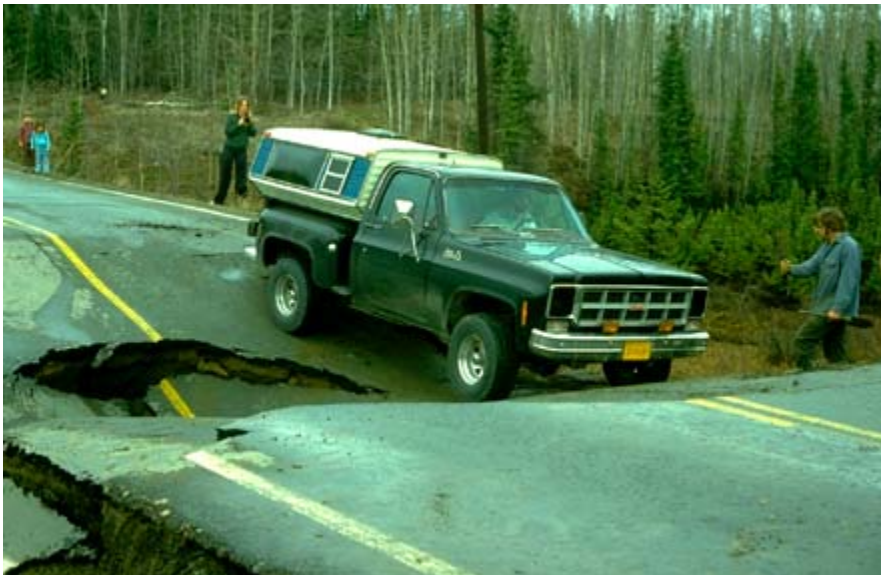
Figure 4.—Collapse of a section of the Alaska Highway in 1982 resulting from melting of massive ice under the roadbed. (Photo by Joe Moore, USDA, NRCS.)
