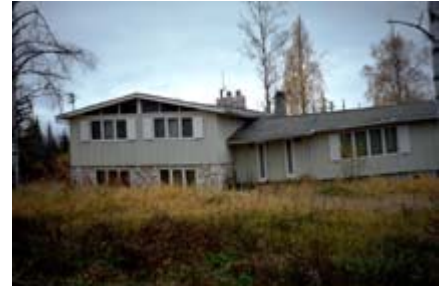
Figure 5.—The result of building a conventional foundation on permafrost-affected soils containing massive ice. Heat transfer from the house resulted in melting of the ice and displacement of the foundation.
