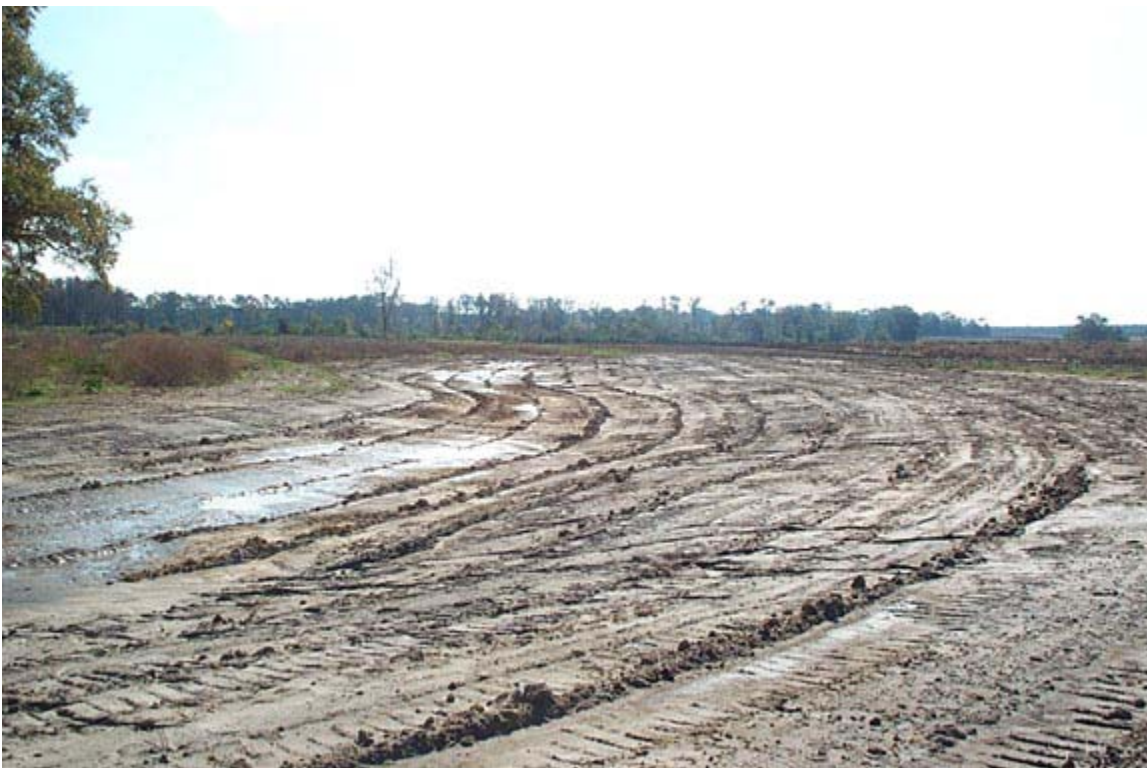
Newly constructed crescent shaped swale adjacent to the end of an existing hedgerow.
