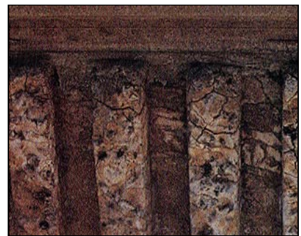
Figure 3. A close-up view of the panel in Figure 2 shows cracked concrete caused by cyclic freezing of inadequately air-entrained concrete.
