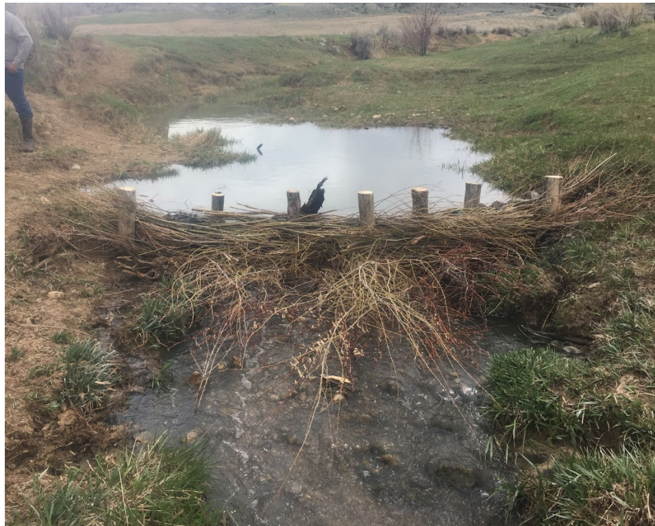
Figure 9: Newly Installed BDA May, 2019
