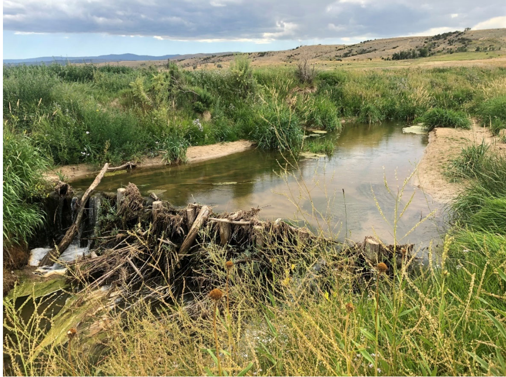
Figure 10: Newly Installed BDA September 5 th , 2019
