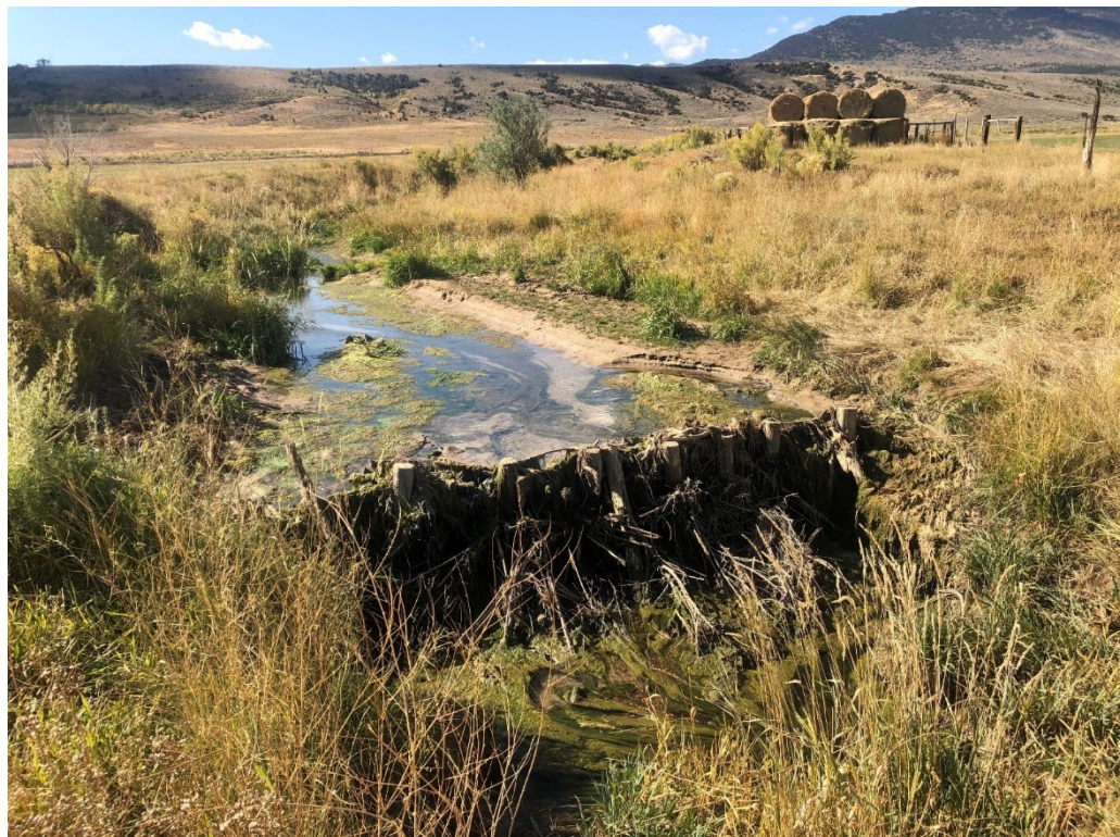
Figure 11: Newly Installed BDA October 4 th , 2019
