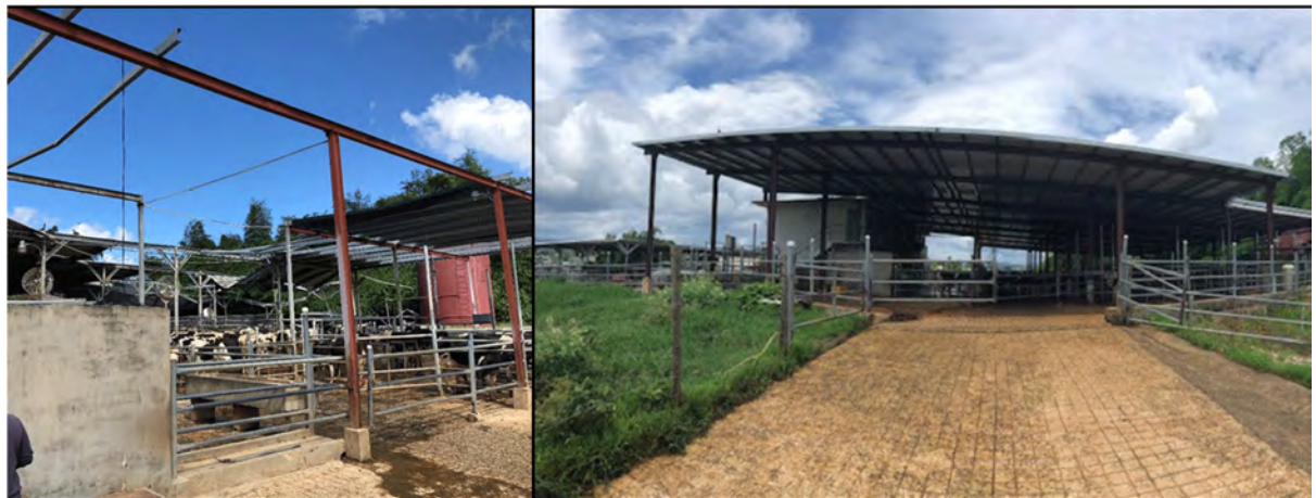
Right: BEFORE—Morovis dairy barn roofs and covers destroyed by Hurricane Maria (Photo from Rafael Davila, Sep. 2018). Far right: AFTER – Cattle safely enclosed after farmer installed 14,000 square feet of NRCS Roofs & Covers practice, built to new stronger standards to withstand higher wind speeds (Oct. 2019).
