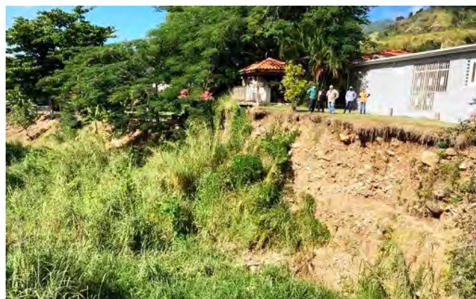
Caribe Soil & Water Conservation District and NRCS EWPP staff hold an on-site kick-off meeting for the first Hurricane María EWPP Structural Stabilization project in Villalba in September 2021.
