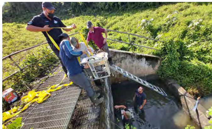
NRCS Engineer Rolando Collazo and contractors from Torres Rosa, Inc., and Freese-Nichols, Inc., inspect the Ajies Dam principal spillway conduit (250' of 30" diameter reinforced concrete pipe) from impact basin to riser across the earthen dam using Remotely Operated Vehicle equipment to visually inspect the internal condition of the pipeline and its joints.
